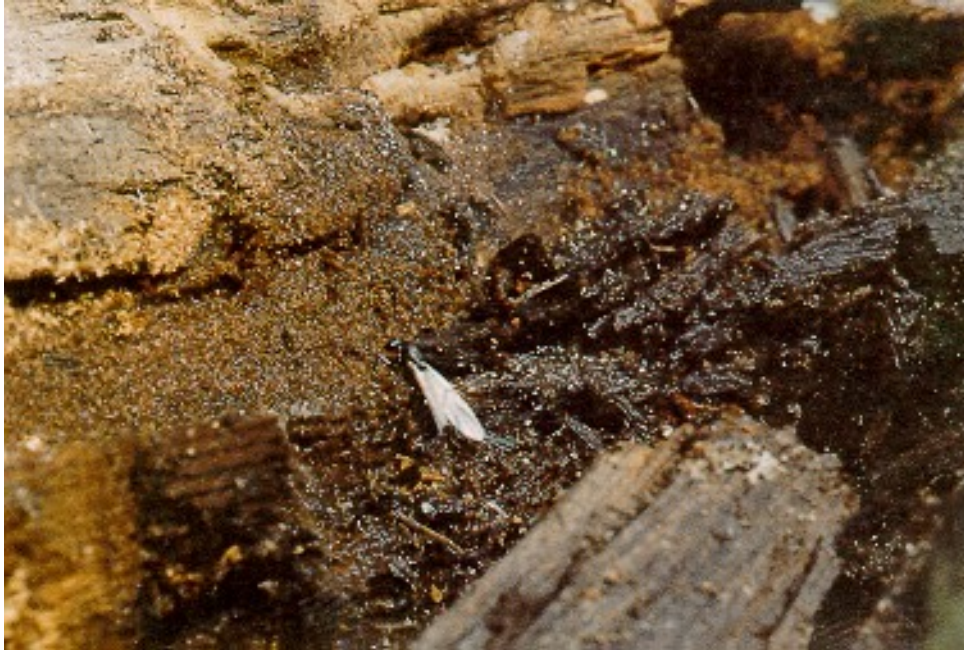
Figure 2.4.3(b) Very Severe Insect Damage in Wood
