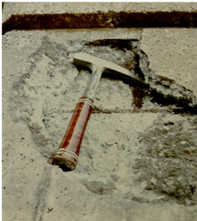
Figure 2.2.6(b) Severe Local Spalling
