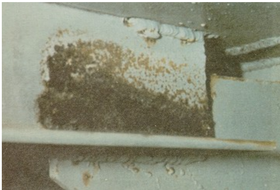
Figure 2.8.1(d) Chemical Attack
