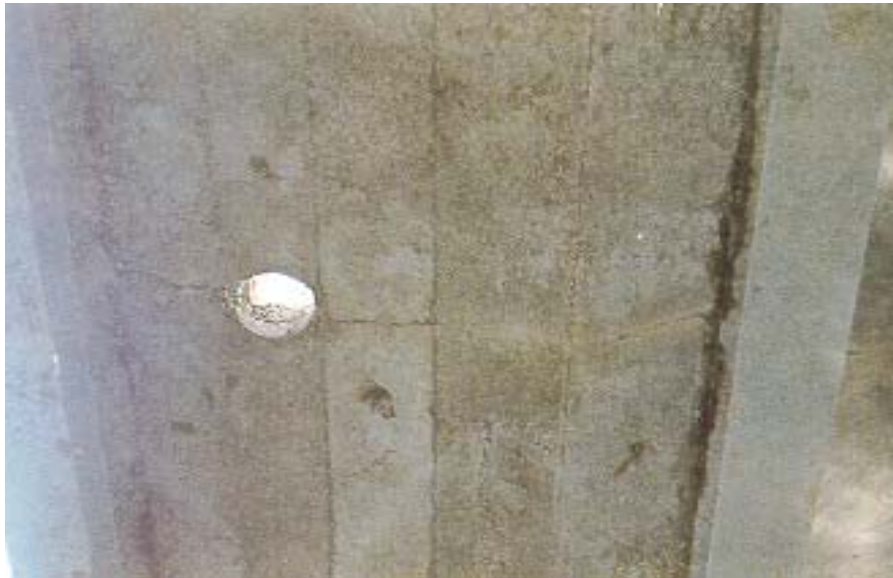
Figure 8.8(e) Deck Drain (Hole in Deck)
