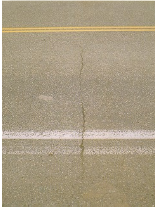
Figure 2.7.1(b) Medium Transverse Crack
