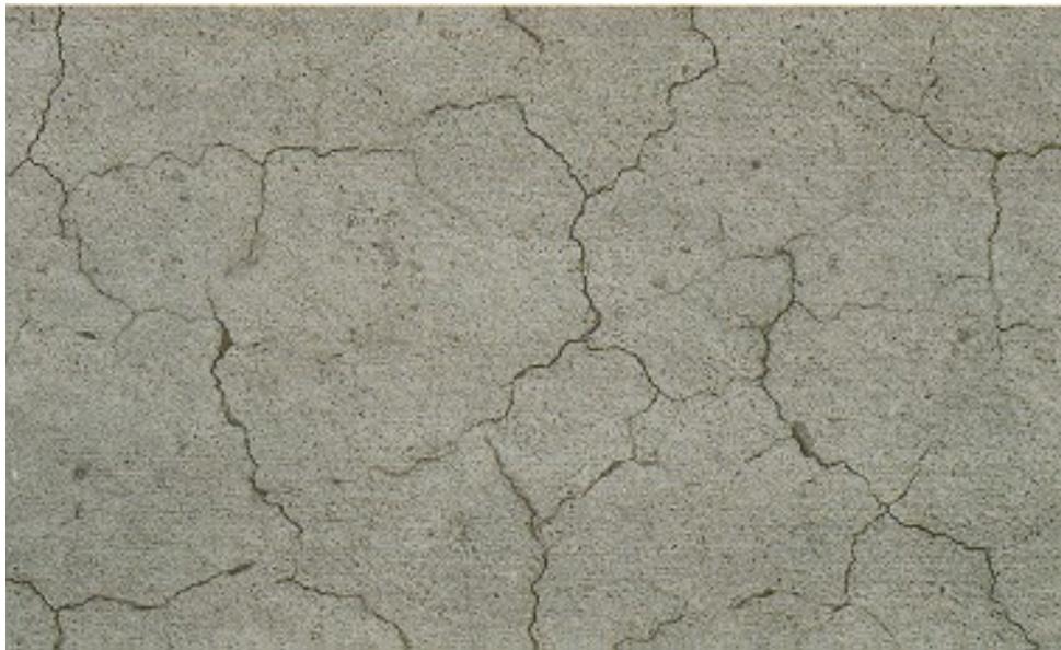
Figure 2.2.8 Severe Alkali-Aggregate Reaction
