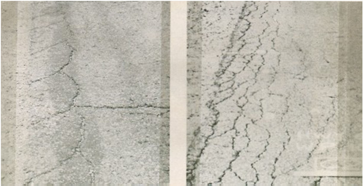
Figure 2.7.1(e) Medium Progressive Edge Cracks
