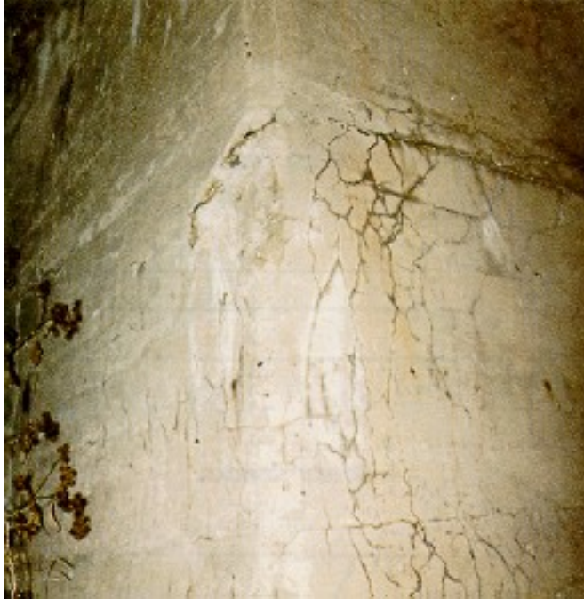
Figure 2.2.7(c) Medium Pattern Cracks in an Abutment
