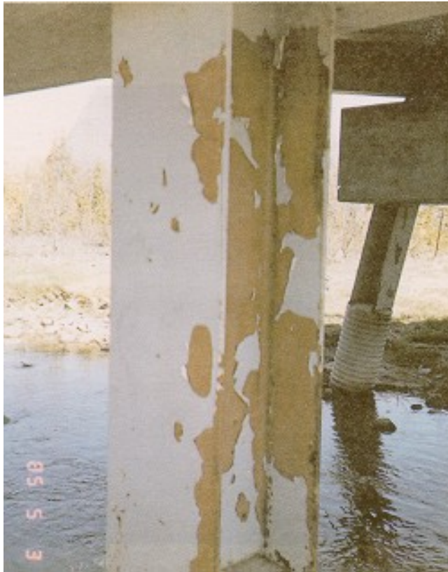
Figure 2.8.2(c) Intercoat Delaminations
