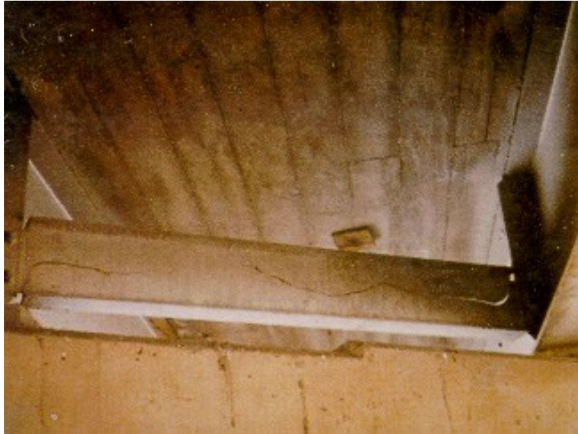
Figure 2.3.3(a) Very Wide Cracks in a Diaphragm
