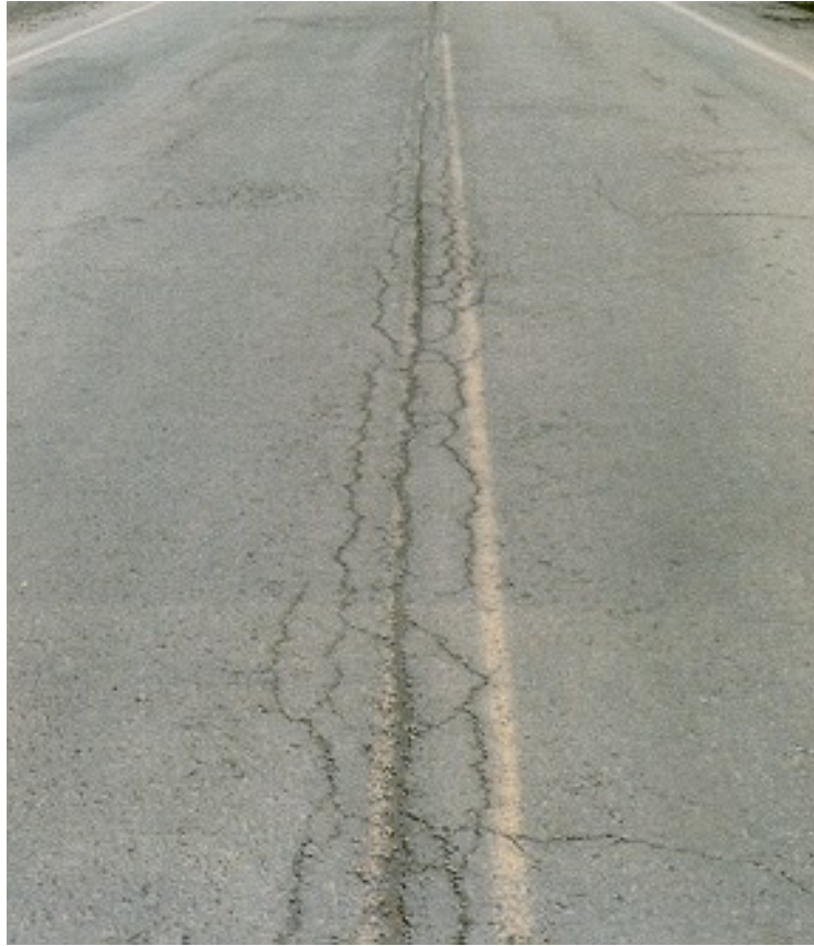
Figure 2.7.1(a) Medium Longitudinal Crack
