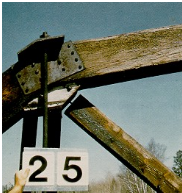
Figure 2.4.7 Loose Connection in Wood (25 mm gap measured)
