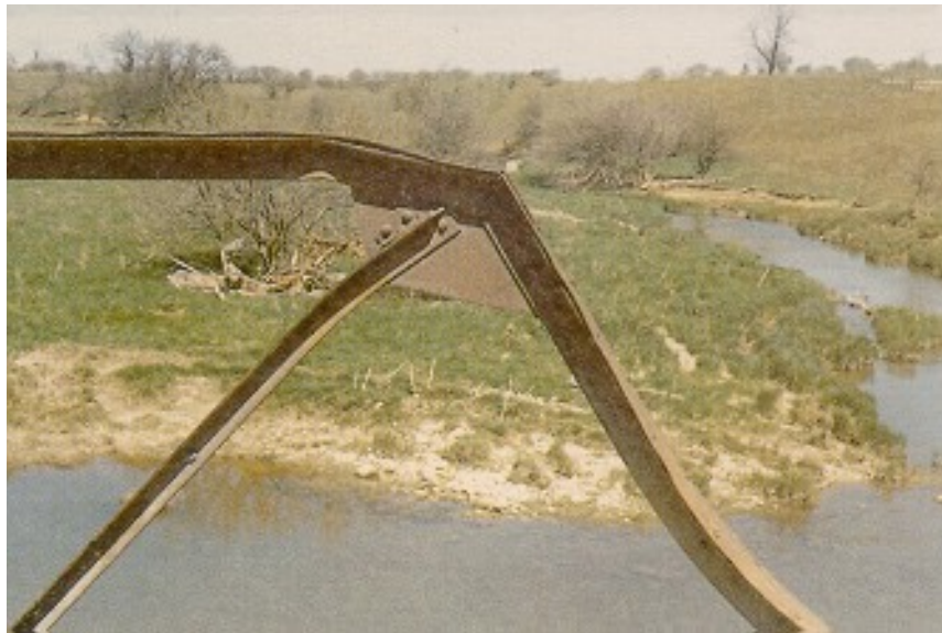
Figure 2.3.2 Very Severe Permanent Deformations by Impact
