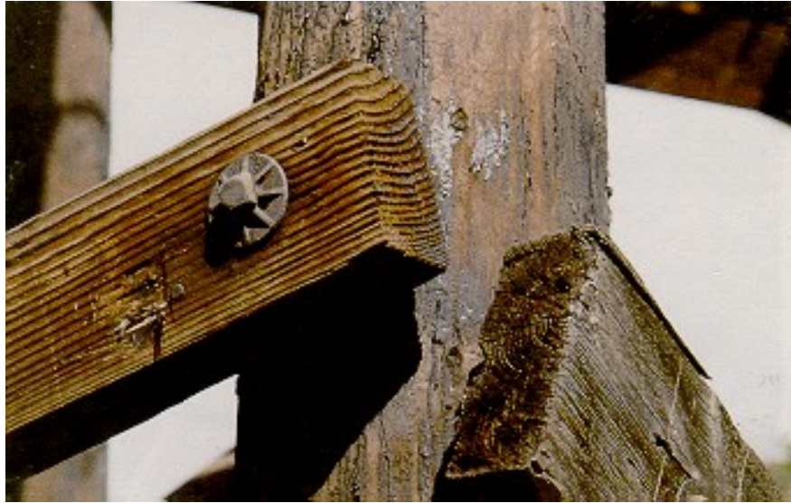
Figure 2.4.1(a) Light Weathering in Wood Members
