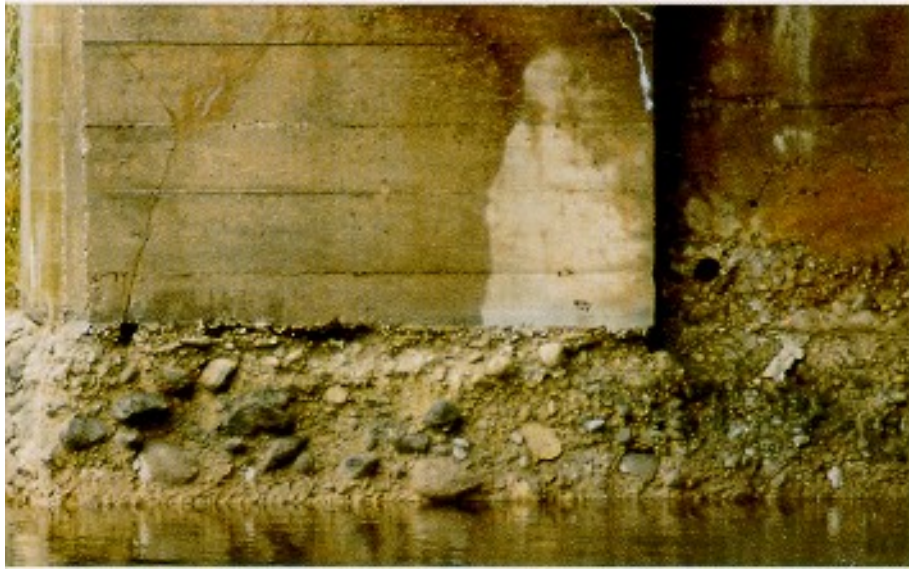
Figure 2.2.3 Very Severe Erosion of a Concrete Footing
