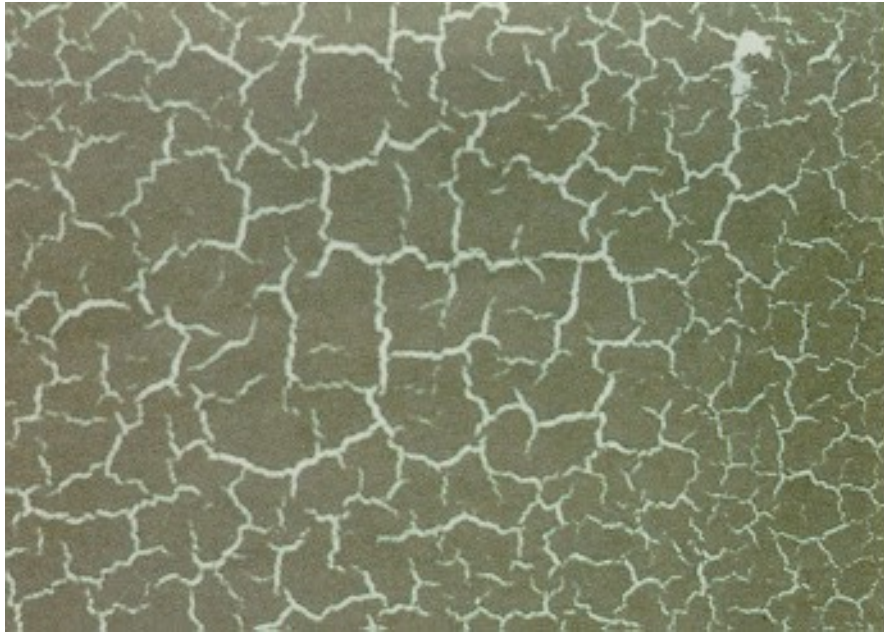
Figure 2.8.1(c) Alligatoring (typical mud crack pattern)
