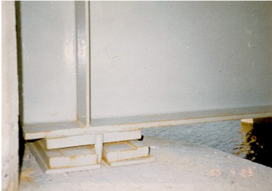
Figure 2.8.3(a) Edge Defects
