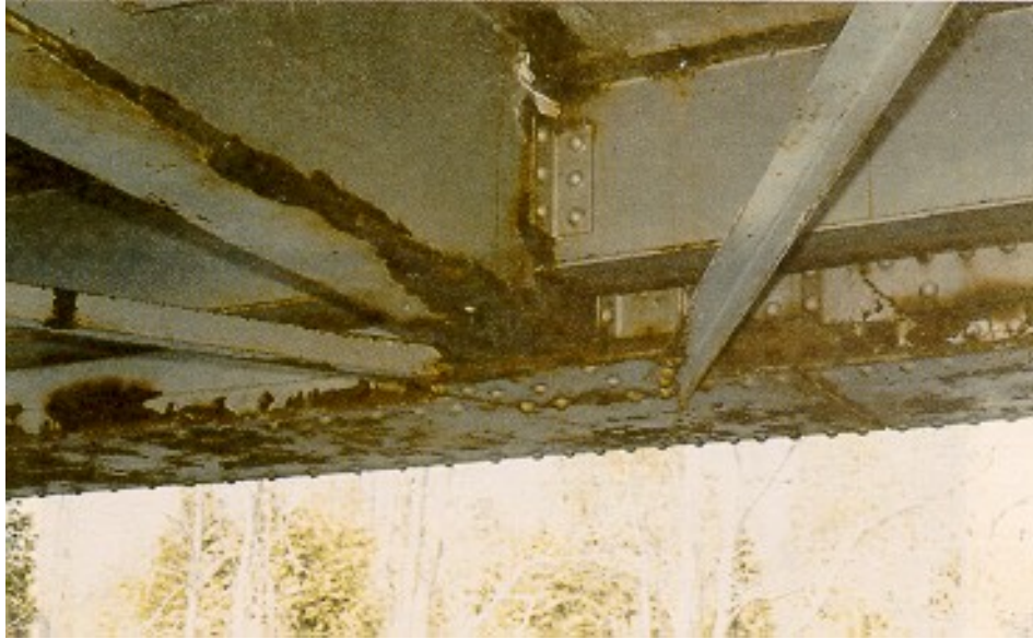
Figure 2.3.1 Medium Corrosion of Steel Beams
