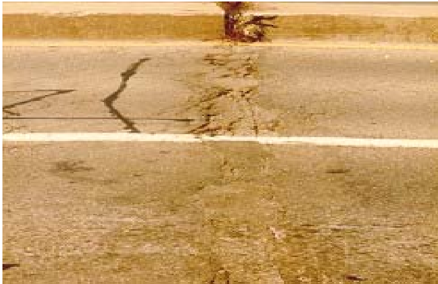
Figure 8.11(c) Paved-Over Joint
