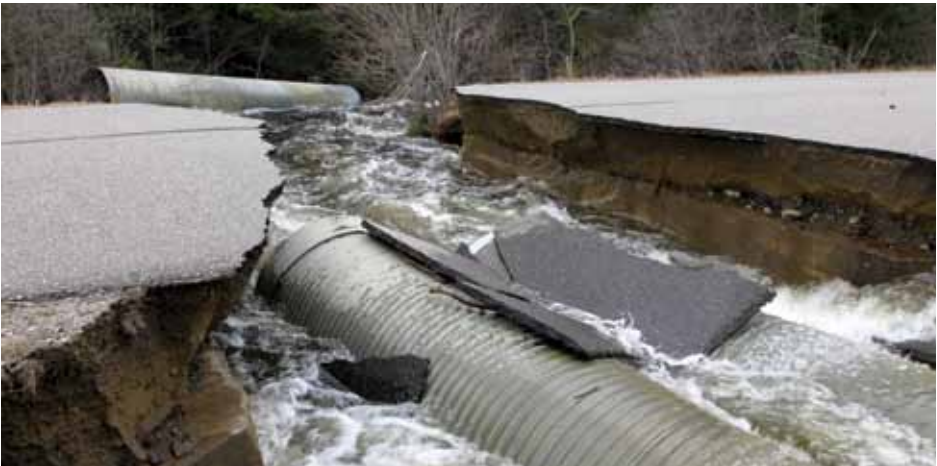
Washout on the Opeongo Road on April 20, 2013.
