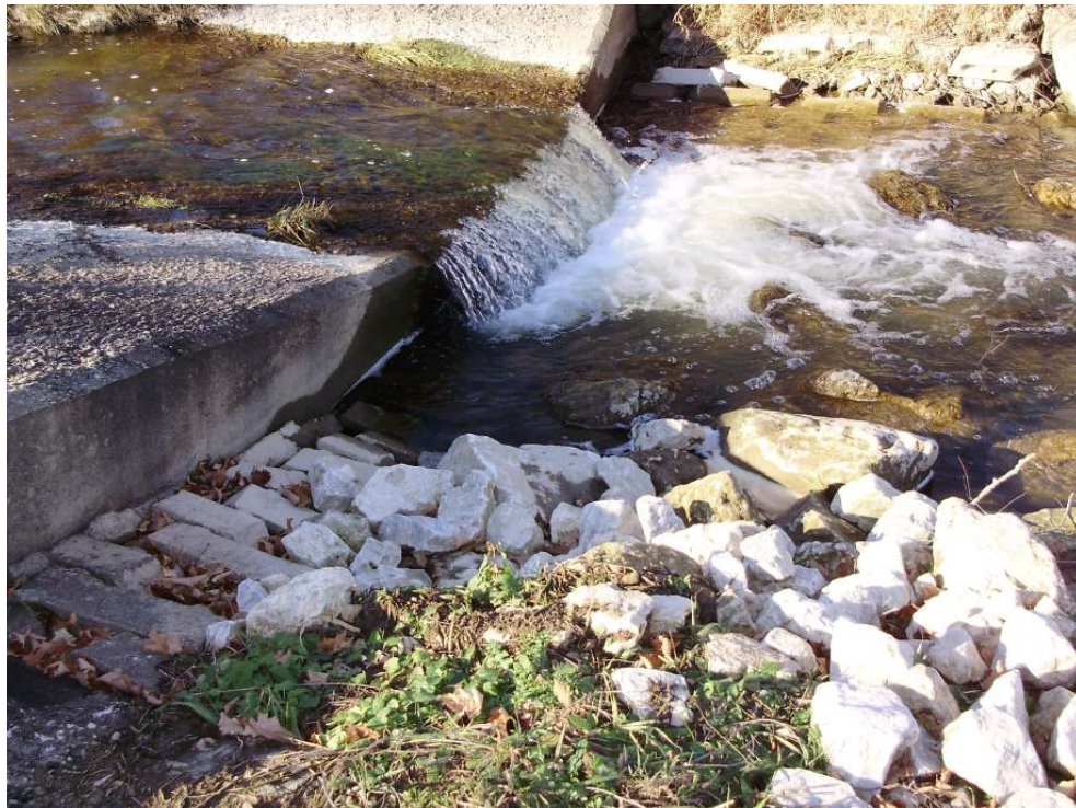
Eroded shoreline at, and downstream of the concrete weir on Willow Creek in Paisley. Repairs were made in 2010.
