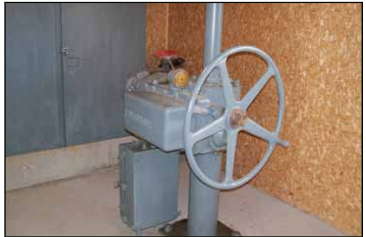
Gate controller for Parkhill Dam.
