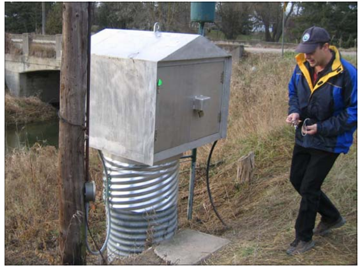
Water Resources Technologist, Brian Smith, at one of the NVCA's gauges, which are used to measure the height of the water in the stream channel. The data is then compared to pre-recorded stream flows.
