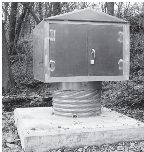
This is a typical stream gauge installation; they are often described as resembling steel dog houses.
