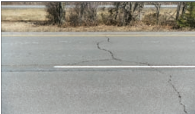
Transverse and longitudinal cracks on Highway 417.
