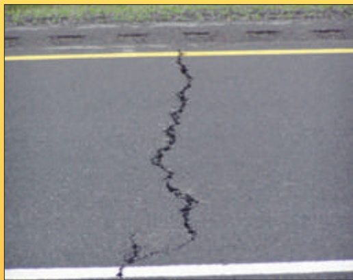
Premature cracking lowers overall pavement performance.
