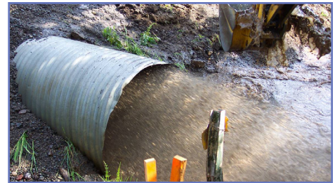
Culvert debris was easily displaced and discharged.
