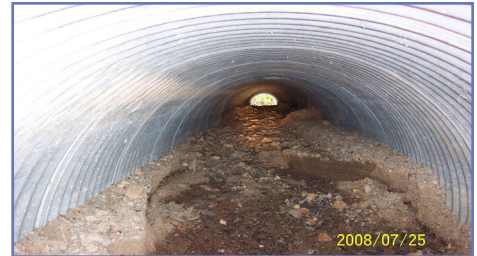
The culvert on Highway 590 filled with gravel and rocks after a June 2008 rain storm.
