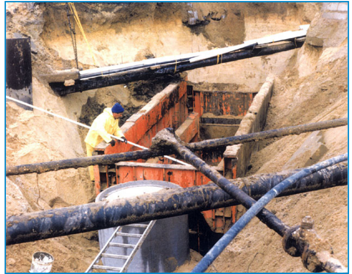
CSA's S250 standard will help utility and road owners get a better handle on underground spaces.
