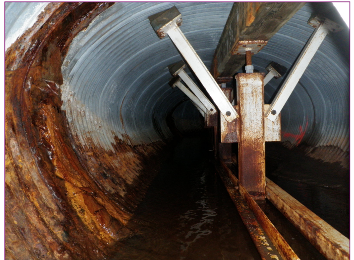
Figure 3: Two sections of the Corrugated Steel Pipe braced in 2009 to prevent further movement.
