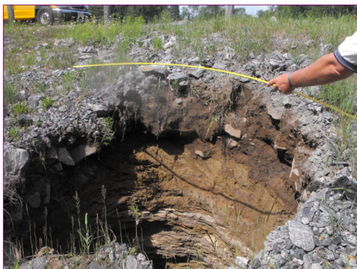
Figure 2: A sinkhole developing in the east embankment threatens the integrity of the adjacent northbound lane on Highway 11.
