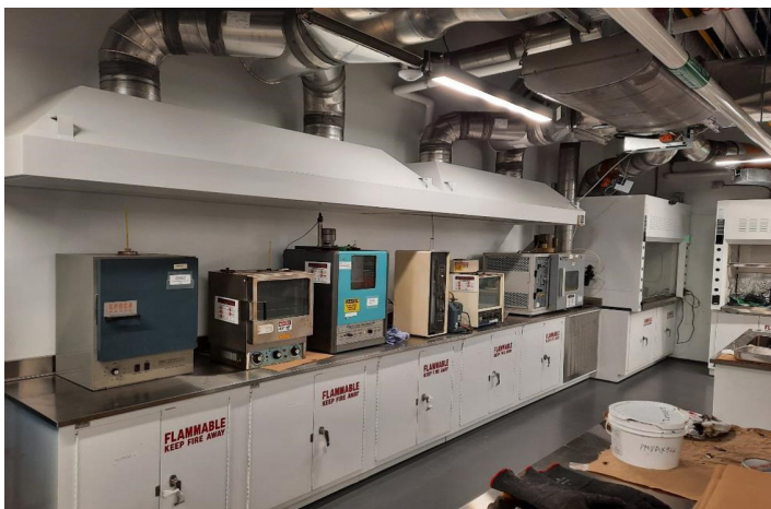
Equipment in the bituminous materials lab.
