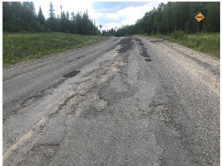
An example of road surface pavement damage.
