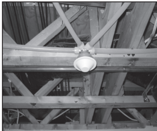
A picture of the sprinkler head and piping in the ceiling before the drywall was installed in the Chief's mechanical room.
