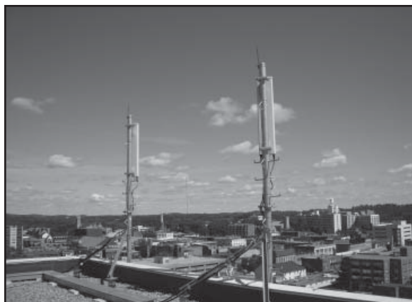
A picture of two lightning rods protecting cellular antennas atop a building.
