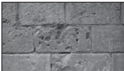
The wall that still bears the evidence of gouged concrete from the fired rounds of a firing squad during WWII.
