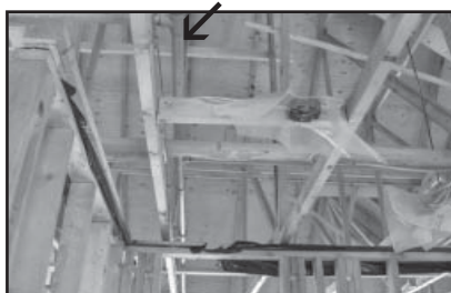
A photo of the sprinkler piping system (see arrow pointing to pipe) before it was concealed with wallboard at Chief Mintz's home.
