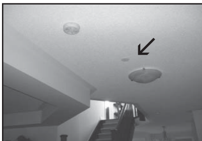
A photo of a ceiling in Chief Beckett's home. Notice how inconspicuous the sprinkler plate is in comparison to the smoke alarm and lighting fixture.
