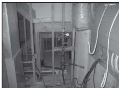
A picture of Mintz's sprinkler manifold riser.
