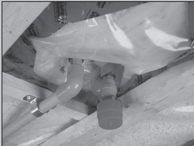
Residential sprinkler piping installed during construction: The red cap protects threads where a sprinkler head will be mounted in ceiling once drywall is installed.
