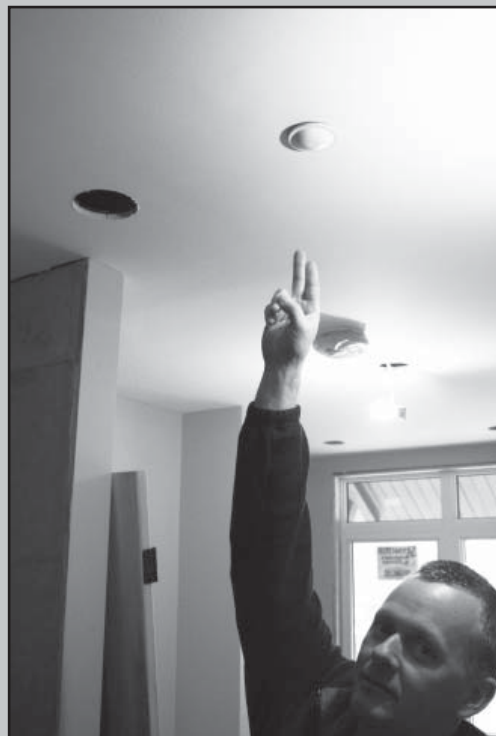
Sprinkler heads can be covered with decorative caps as indicated here by homeowner Terry Ablett.
