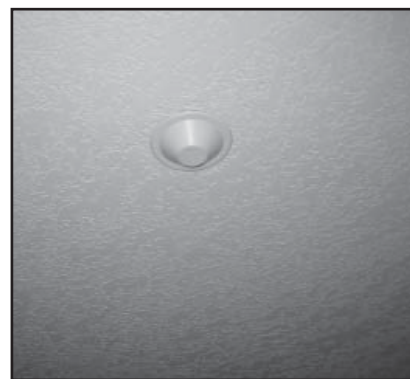
A picture of how one sprinkler system with capped head looks on a home's ceiling.
