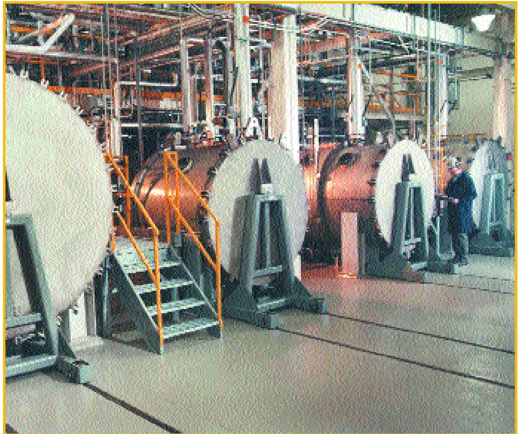
Seen above are the nickel deposition chambers at Weber Manufacturing which are used for the nickel vapour deposition process.
