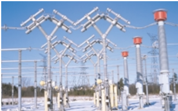
500 kV breakers / Cherrywood TS
