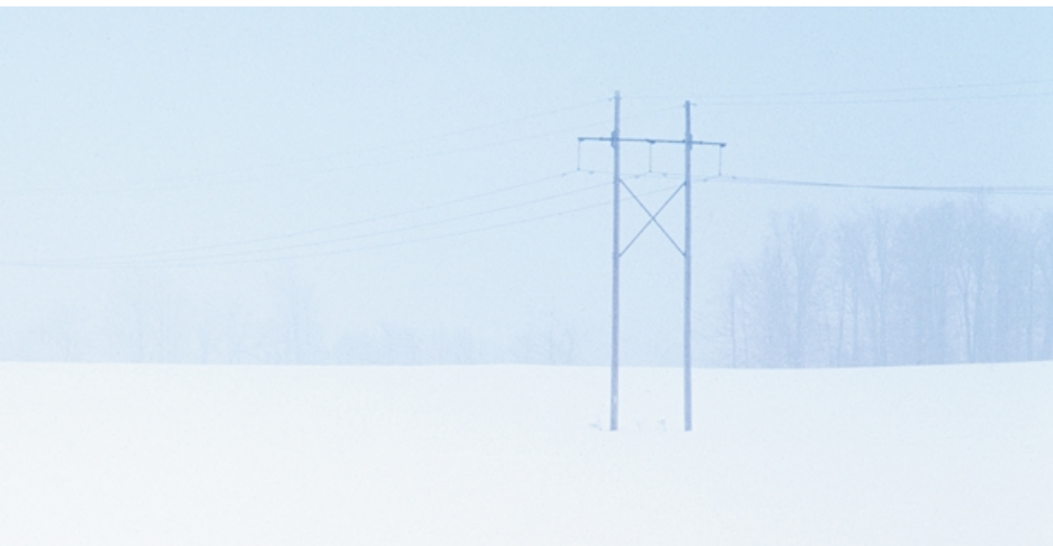
Single circuit H-Frame wood pole structure, 115 kV transmission line / Collingwood, Ontario
