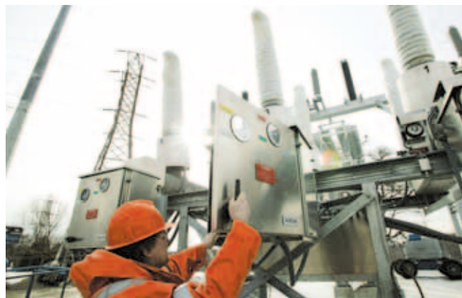
John Wright inspects equipment at our Leaside Transformer Station in Toronto.
