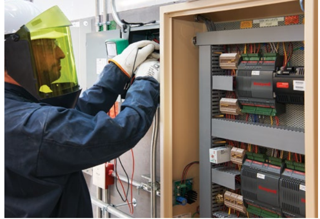
ESA commissioned in-depth behavioural research to better understand how electricians like Curtis Landry of Plan Group make decisions about working on energized equipment and to identify ways to help them get the job done safely.
