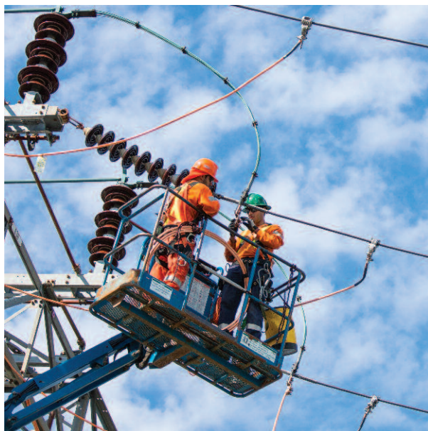
HYDRO ONE NETWORKS INC.
