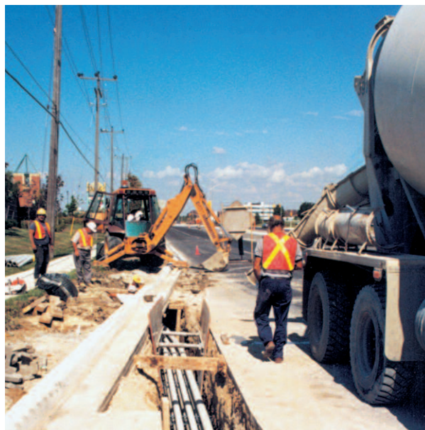
HYDRO ONE BRAMPTON NETWORKS INC.
