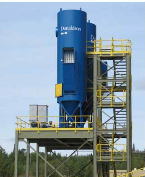
Dust collectors at Atikokan Generating Station
