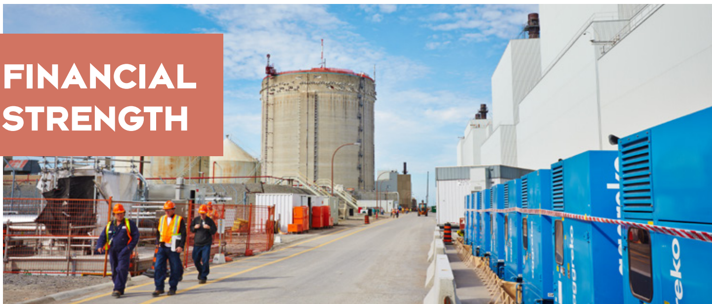
Darlington Nuclear during the Vacuum Building Outage.
