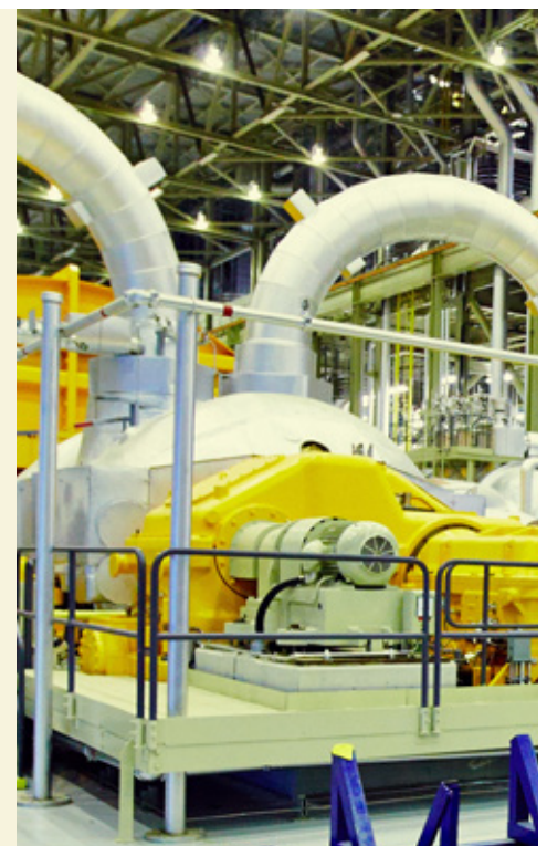
Darlington Nuclear turbine hall.
