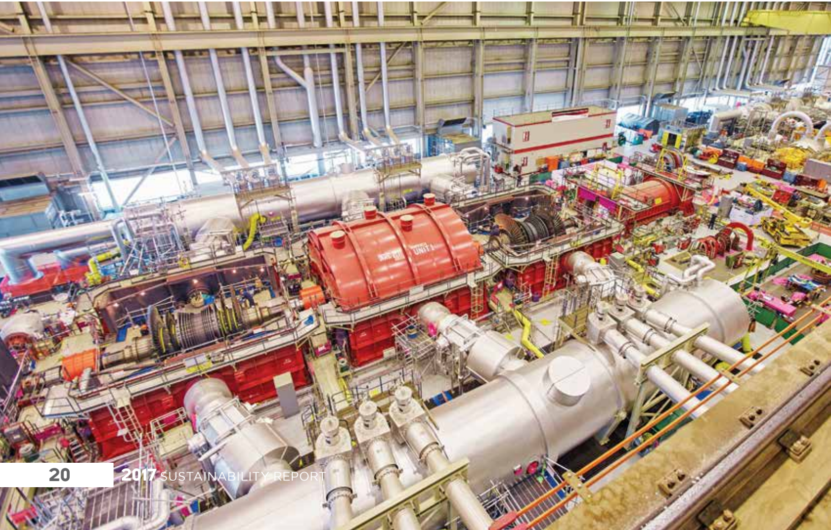
Darlington Nuclear GS turbine hall.
