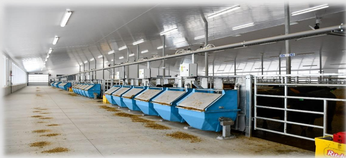
Insentec digital feeders and alley way in the new Ontario Beef Research Centre – Elora.
