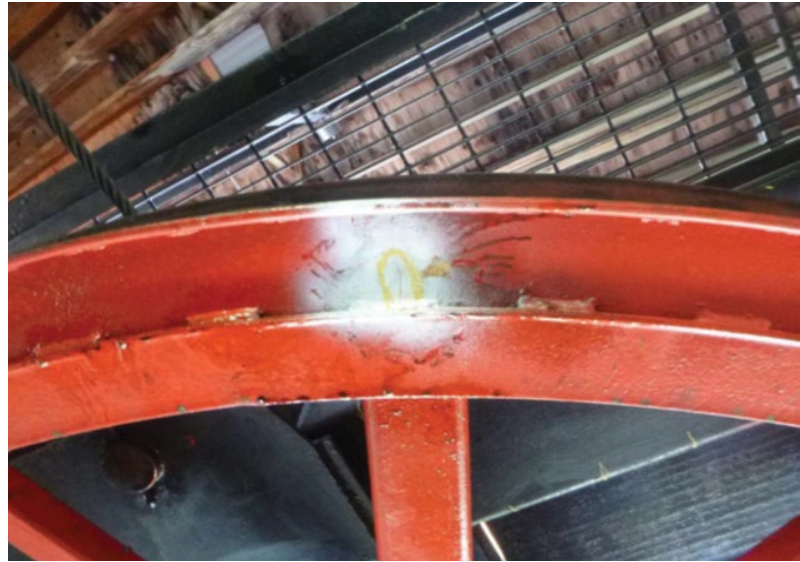
Figure 24: Crack in Bullwheels
