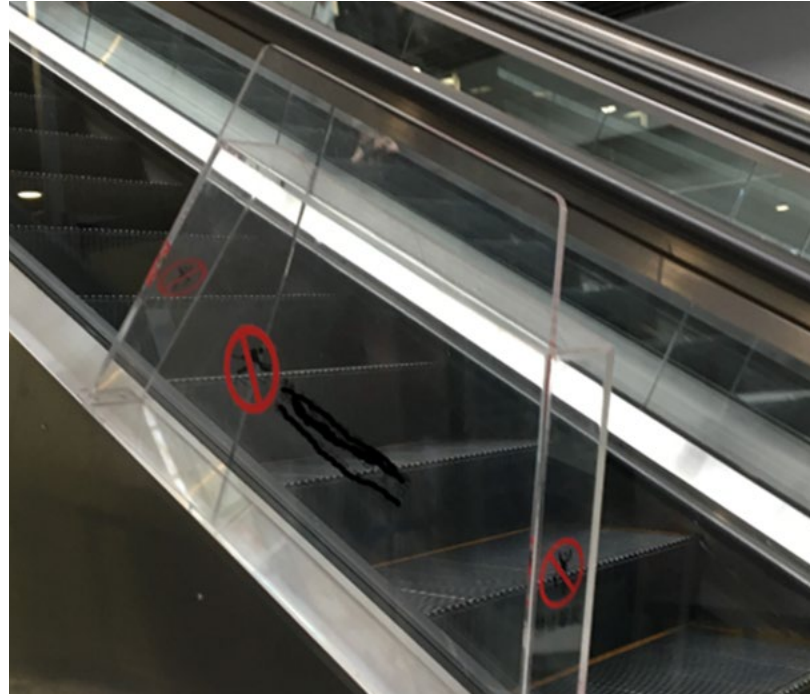
Figure 21: Escalator Deck Barricade
