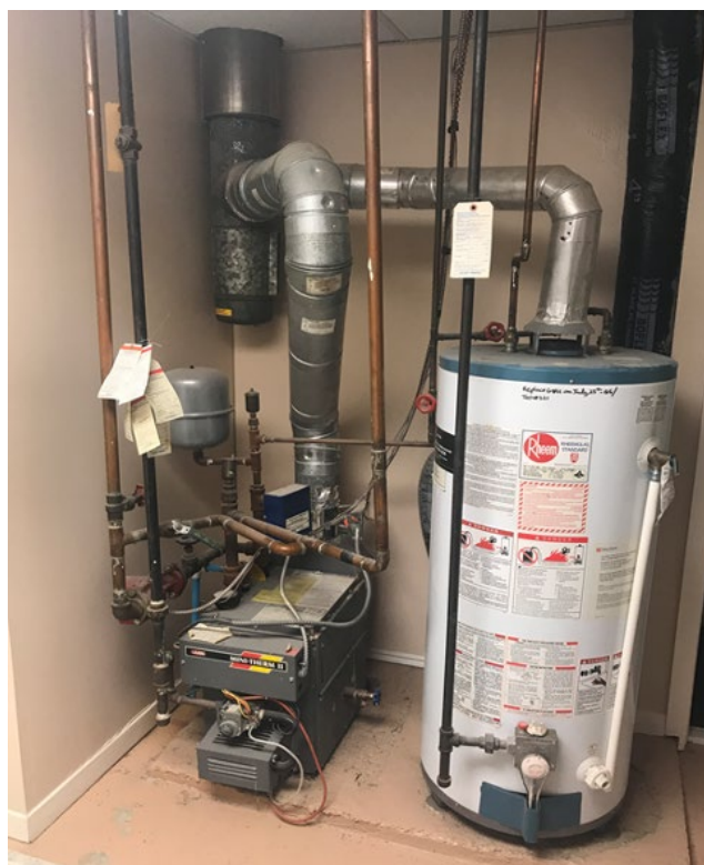
Figure 29: Boiler and Water Heater
