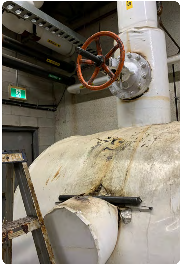
Poorly insulated accumulator steam line
