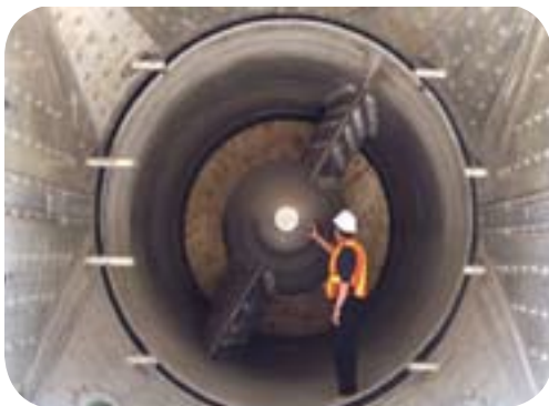
Ted Baldwin, Greenfield Energy Centre's general manager examines the exhaust end of a 200 MW Combustion Turbine.
