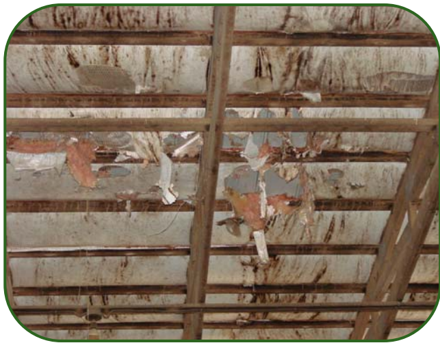
Figure 3. Birds and rodents will damage unprotected insulation
