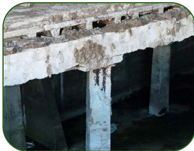
Figure 2. Slats, beams and posts deteriorate when exposed to manure gases
