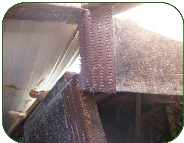
Figure 1. Gusset plates deteriorate with moisture and time
