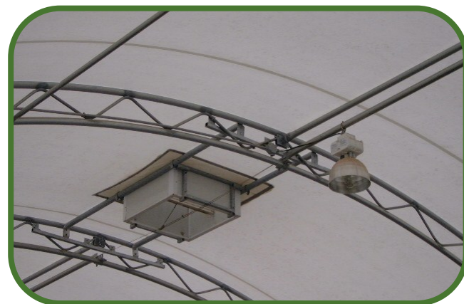
Figure 2. Chimneys for exhausting stale air
