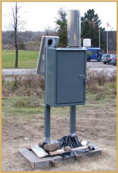
Precipitation water monitoring station.
