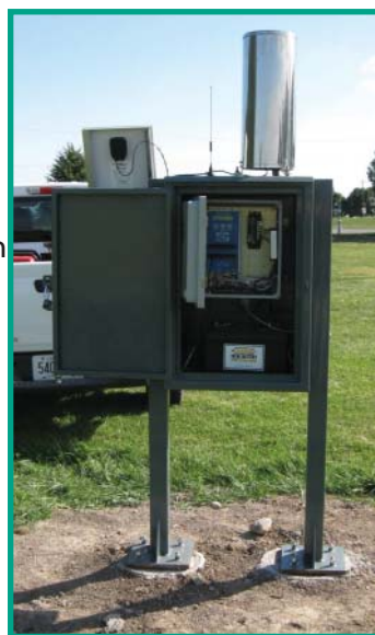
Precipitation water monitoring station.
