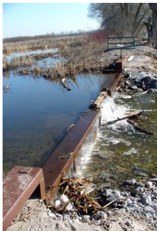
Cranberry Marsh water control structure
