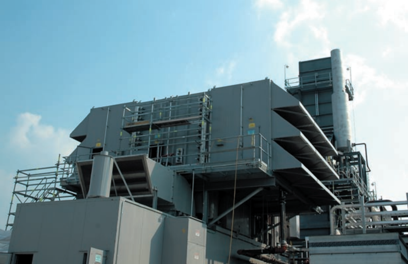
Greater Toronto Airports Authority cogeneration facility
