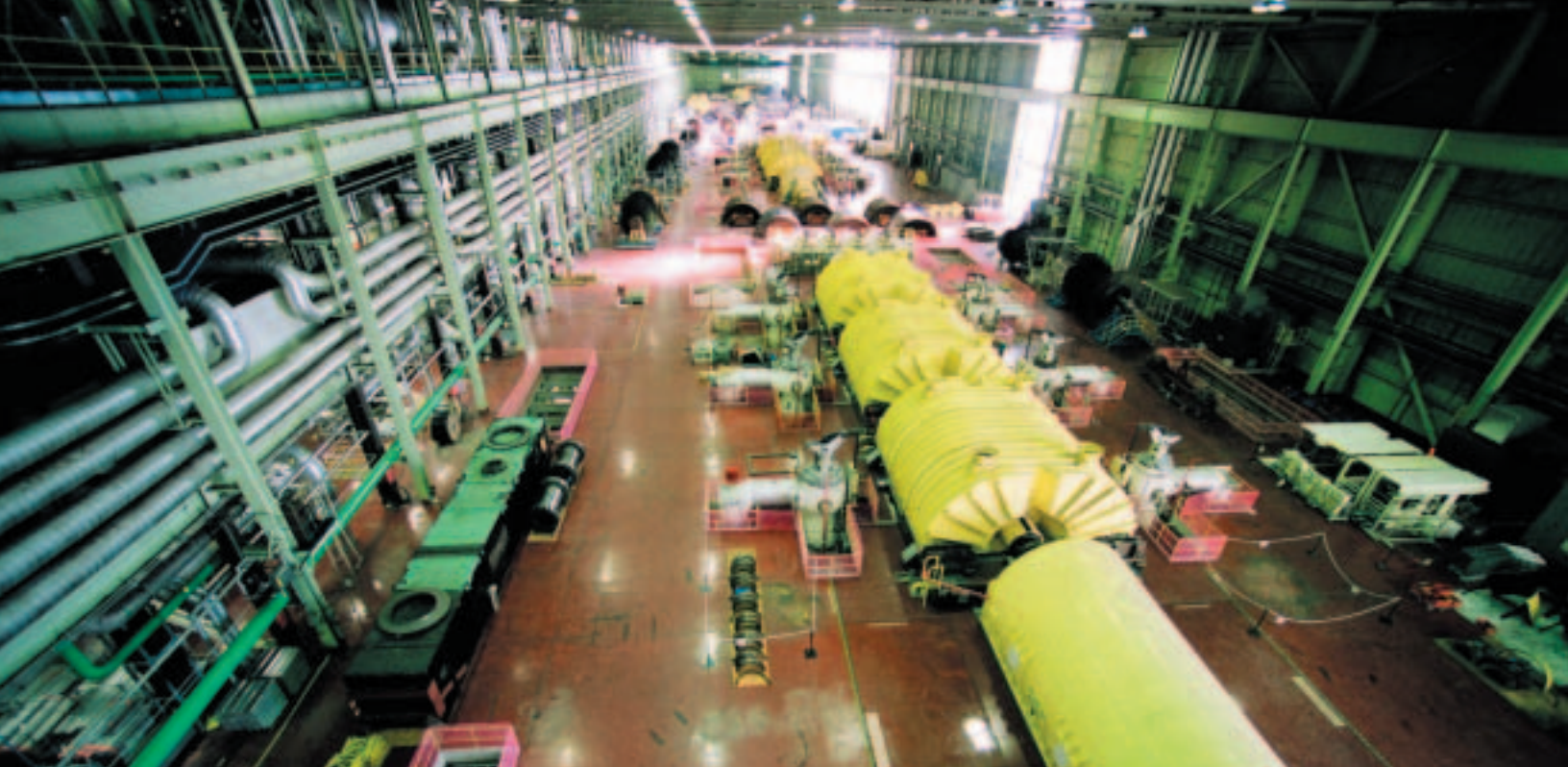
Bruce A Turbine Hall Photo: Bruce Power
