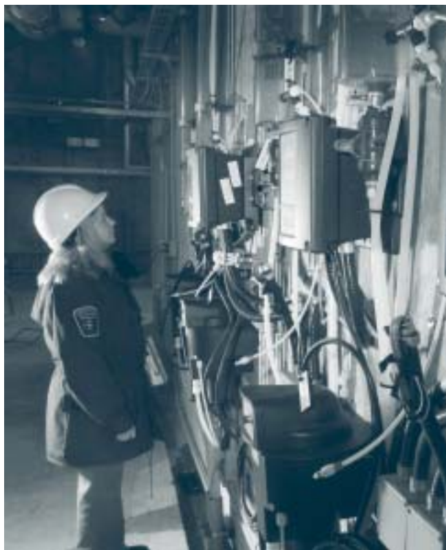
Inspecting digital display of continuous monitoring equipment
