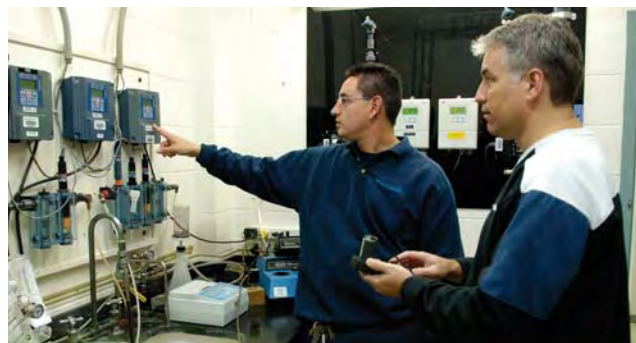
Operators view an on-line chlorine residual monitor.
