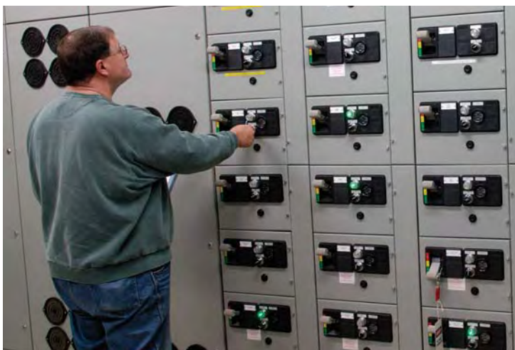
An operator working at the motor control panel in a drinking water treatment plant.
