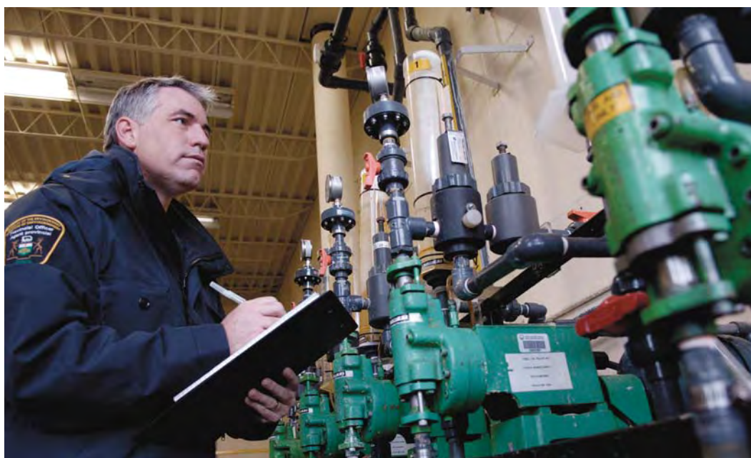
An inspector checking if a chemical (aluminum sulphate or "alum") pump is supplying the proper dosage.
