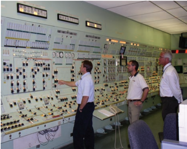
Pickering A Control Room staff synchronize the Unit 1 reactor to the grid for the first time in almost eight years.
