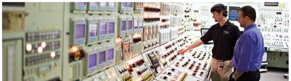
Pickering Nuclear Control Room
