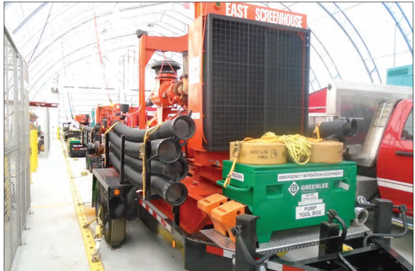
Pickering Nuclear Emergency Mitigating Equipment - diesel pumps and generators.
