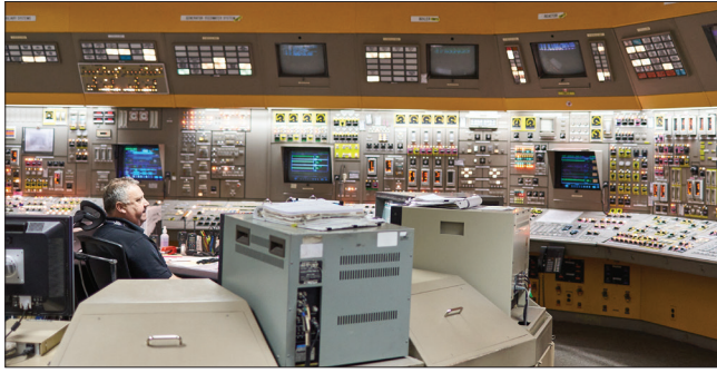
Operator at Control Room Panels
