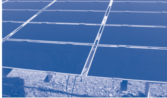
Solar panels at First Light Solar Park.
