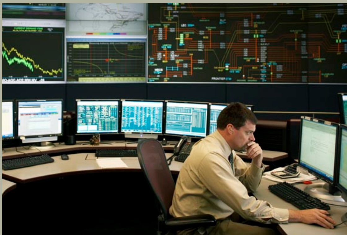
IESO Control Room
