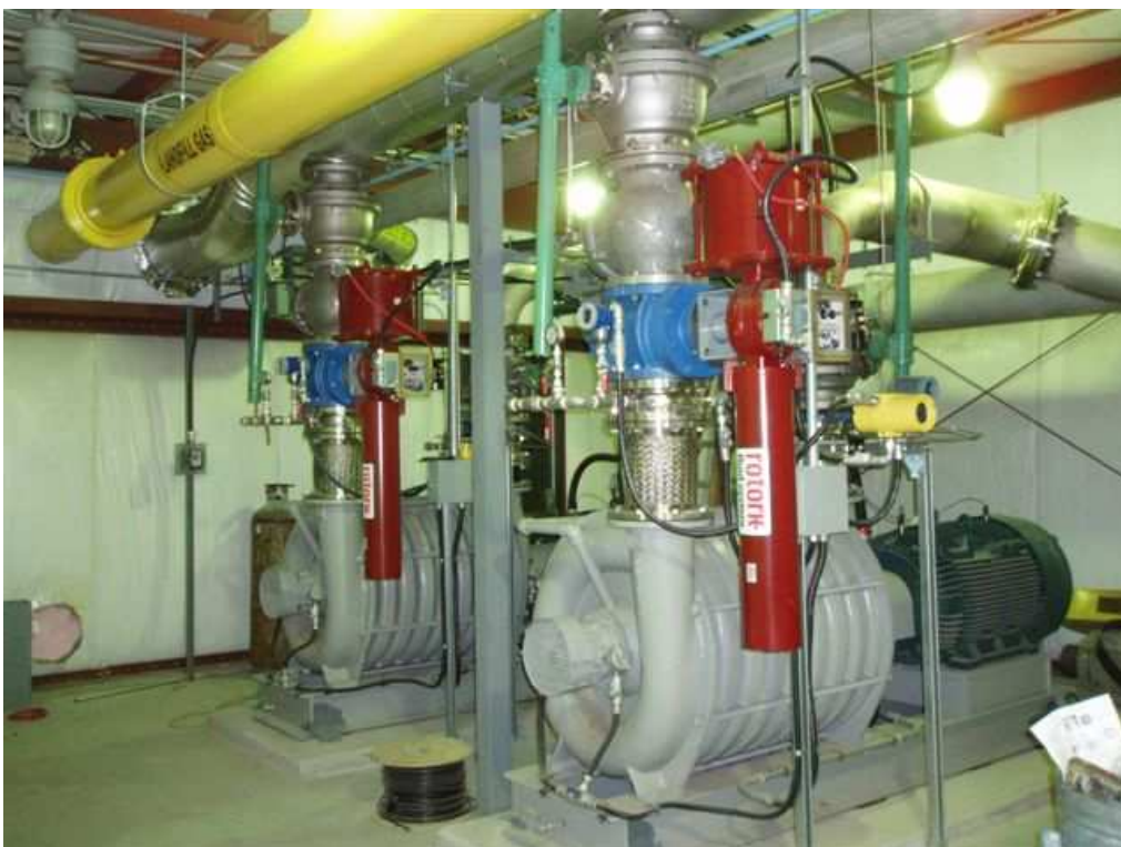
A close up of landfill gas blowers installed at the Trail Road facility.
