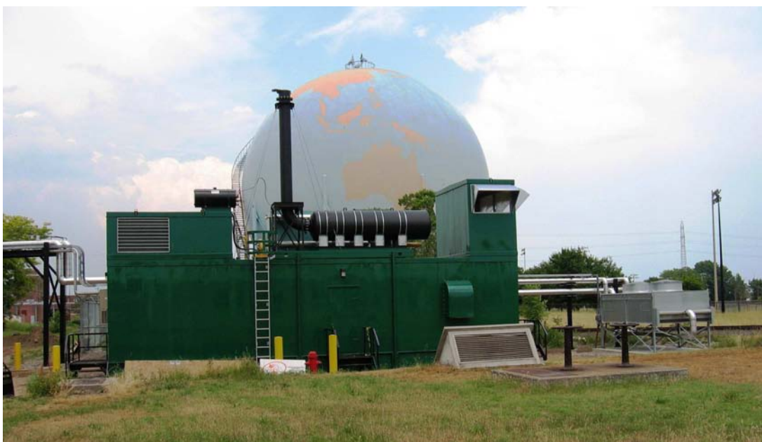
This 1.6 MW digester gas generating facility in Hamilton is the smallest OPA-contracted facility. The project, which was placed in commercial operation in July 2006, was developed by Hamilton Renewable Power Inc., a subsidiary of the City of Hamilton.
