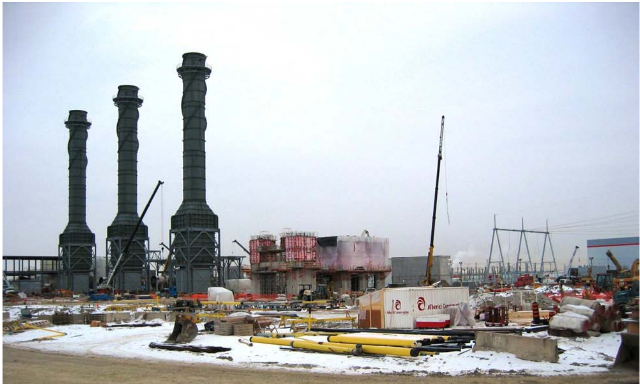
Three by-pass stacks for simple cycle operation have been installed at Goreway.
