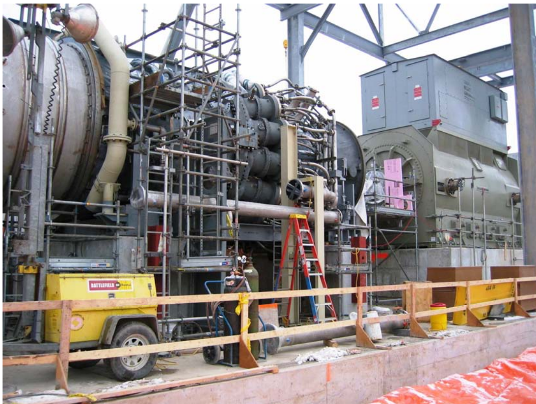
A view of the combustion turbine generator set at Goreway
