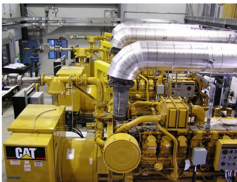
The engine room of the Ecotricity Facility.
