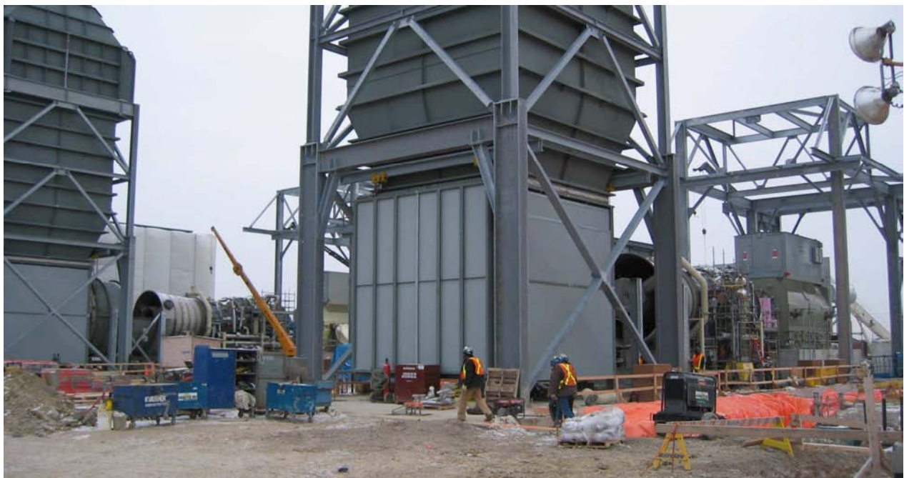
Two of the three combustion turbine generator sets installed at Goreway
