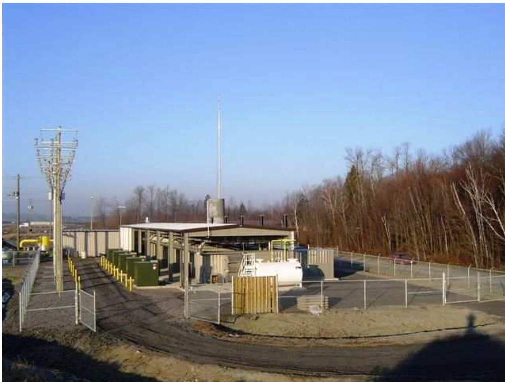
Trail Road is a five MW landfill gas generating facility near Ottawa. The five-unit facility was placed in commercial operation in January 2007. The project was developed by Energy Ottawa.
