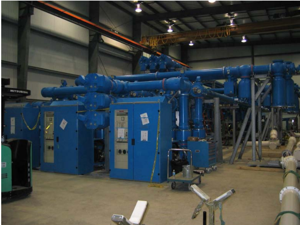
Gas insulation switchgear (GIS) equipment installed inside the GIS Building at Goreway
