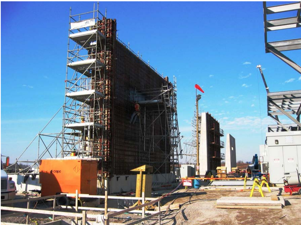
A blast wall for transformer bays installed at GEC
