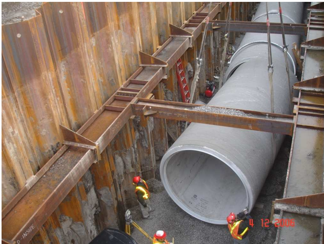
Circulating cooling water pipes are installed at PEC.
