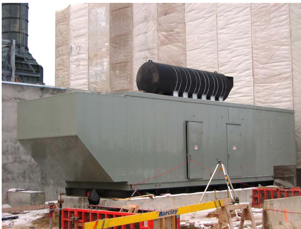
An emergency generator set at Goreway
