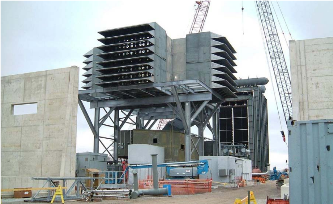
An air intake structure for a combustion turbine installed at GEC
