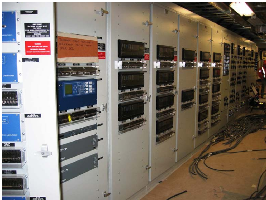
GIS control equipment installed at the GIS Control Room at Goreway
