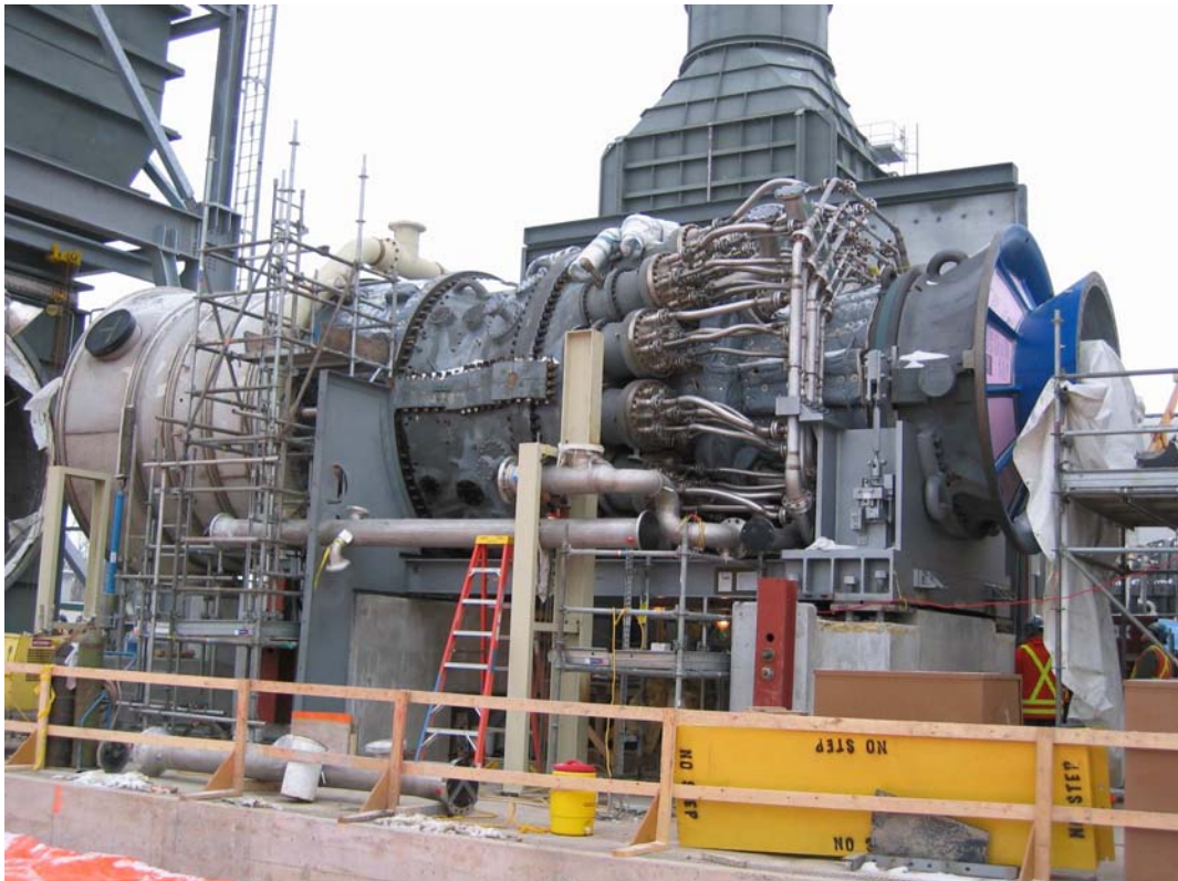
A close-up of the GE 7FB combustion turbine at Goreway
