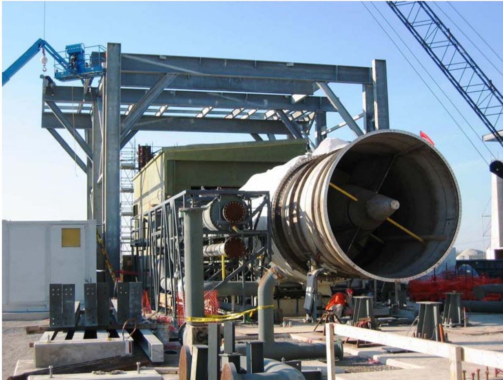
One of the three Siemens Westinghouse F class combustion turbines installed at GEC
