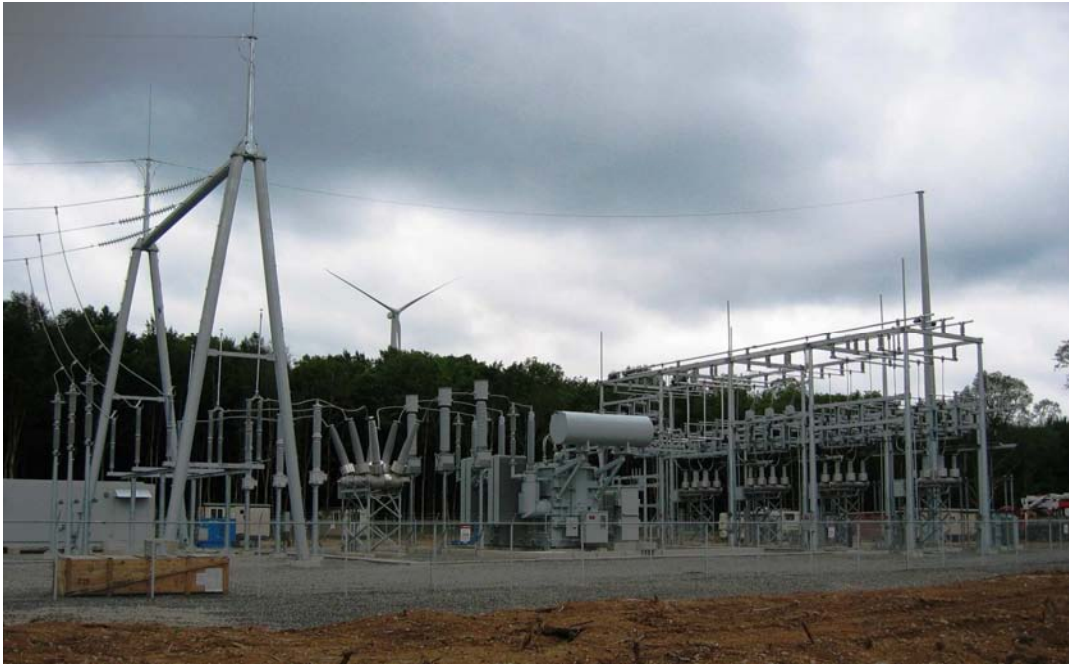
This 34.5/230 kV switchyard steps up the low-voltage energy generated at the Prince Wind Farm for injection into the IESO-administered grid via the Great Lake Power transmission system.
