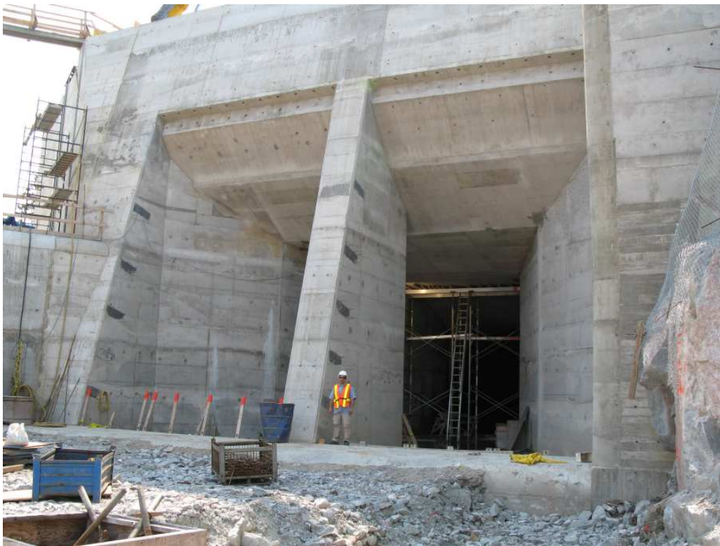
Umbata Falls Hydroelectric Station intake
