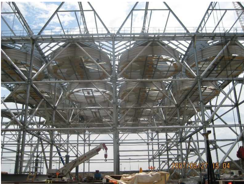
Air cooled condenser area fan assembly
