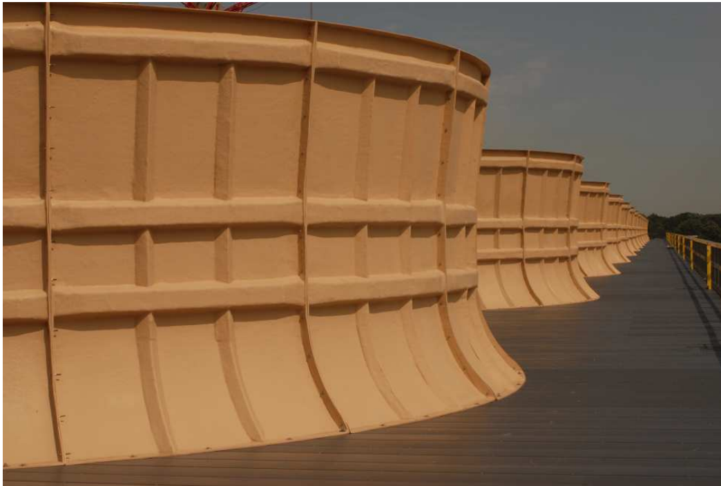
Cooling Towers at Greenfield Energy Centre
