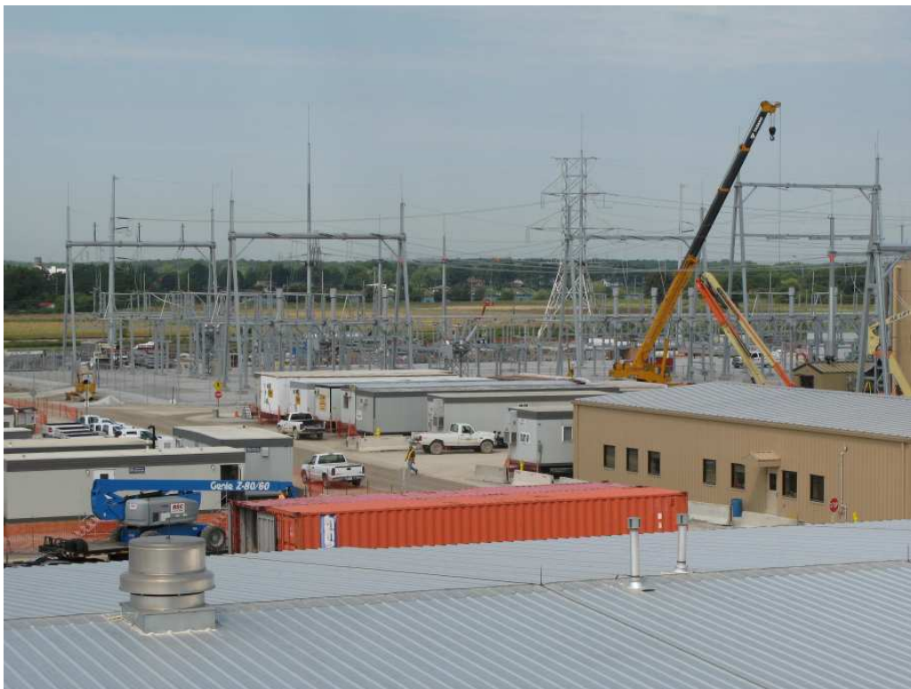
The substation of the Greenfield Energy Centre is close to completion
