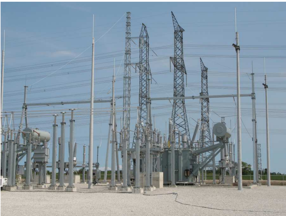
The "north" substation, which is approximately 26 kilometres (km) north of the "south" substation and is located adjacent to Hydro One's 230kV circuits
