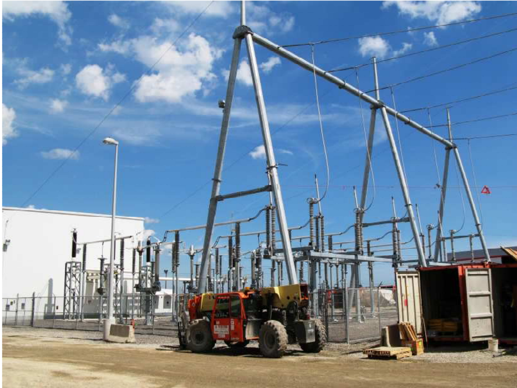
Substation at Goreway Station close to completion
