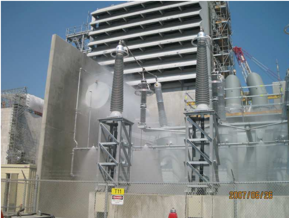
Deluge testing one of the generator step-up transformers at Goreway Station
