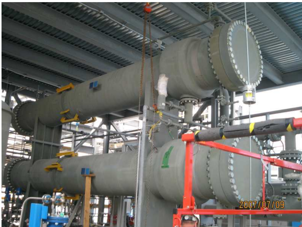
Fuel gas heat exchange at Goreway Station
