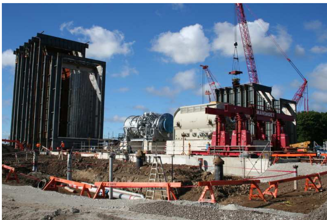
One of the two GE 7FA combustion turbine generators set on pedestals at the St Clair Energy Centre
