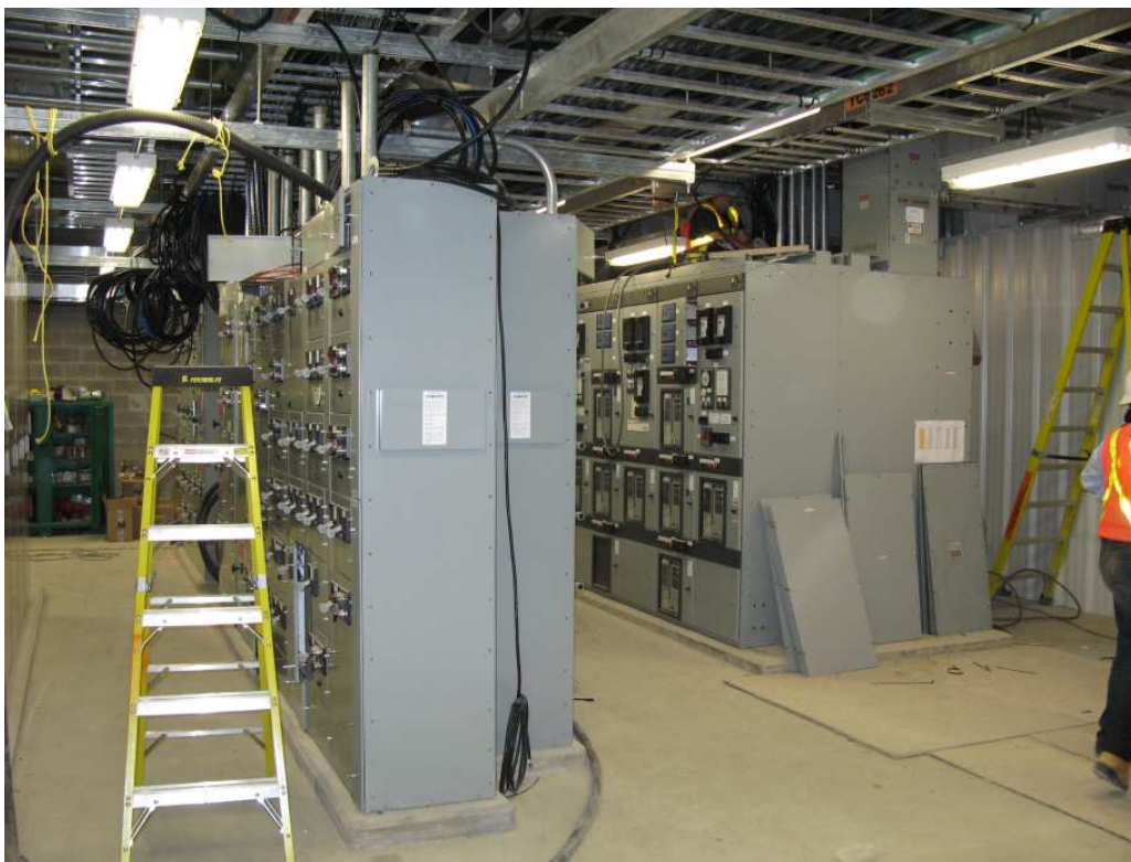
A view of the electrical installation at Greenfield Energy Centre
