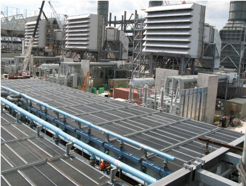
Fin fan area at Goreway Station
