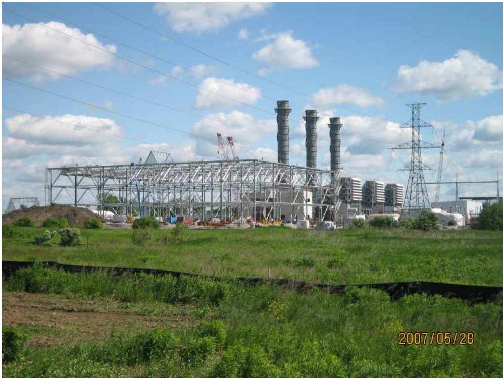
West view of the 860 MW Goreway Station at Brampton; the station adopted a "3-on-1" configuration with three GE 7FB combustion turbine generators, three heat recovery steam generators and one steam turbine generator
