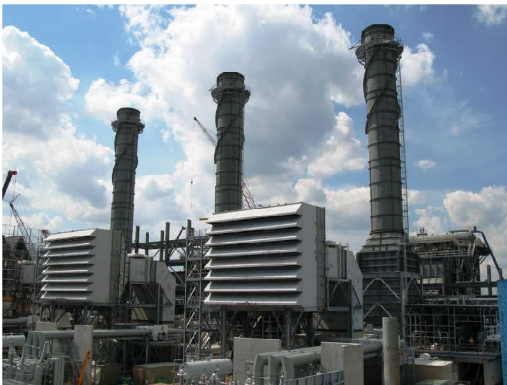
A view of the combustion turbine generator air intakes and by-pass stacks at Goreway Station
