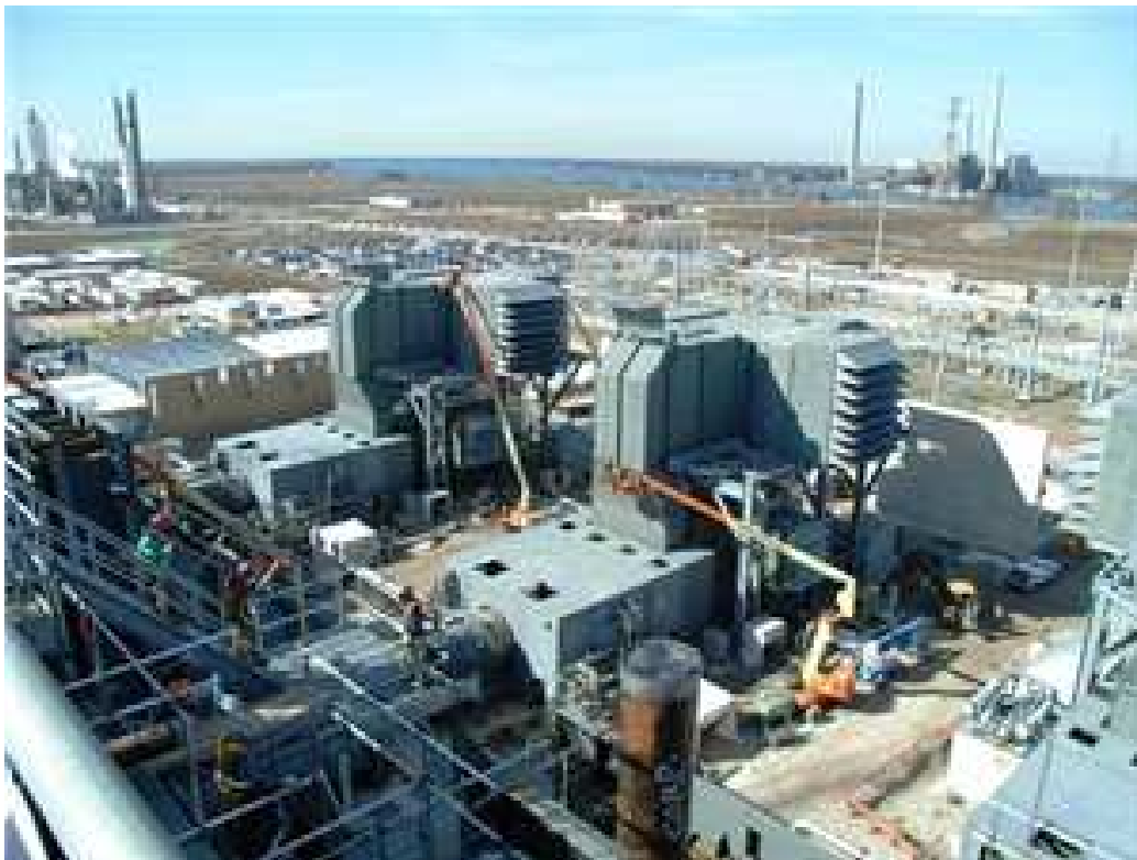
Two of three combustion turbine generator sets at Greenfield Energy Centre
