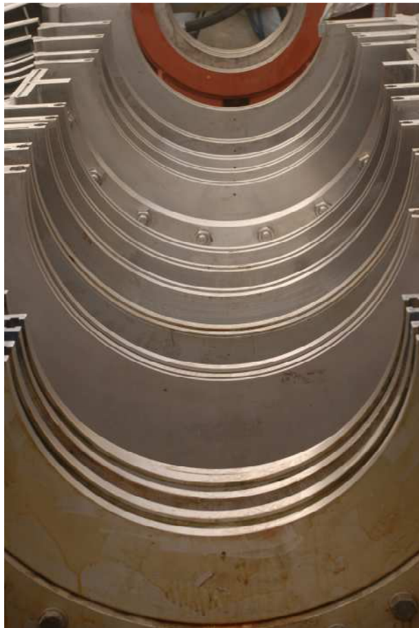
Another view of steam turbine casing at Greenfield Energy Centre
