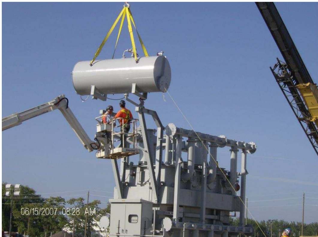
Generator step-up transformer assembly at Portlands
