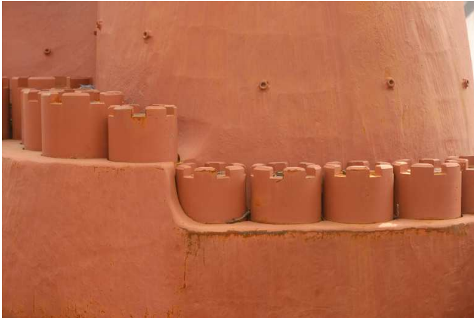
Close-up of IP turbine casing at Greenfield Energy Centre
