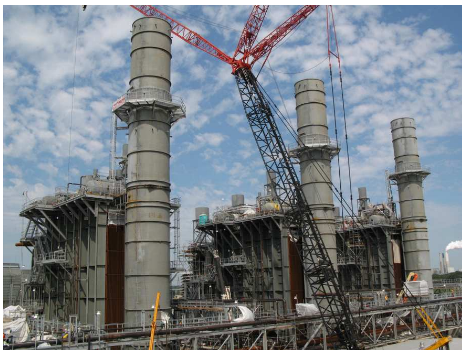
Heat Recovery Steam Generators and stacks at Greenfield Energy Centre
