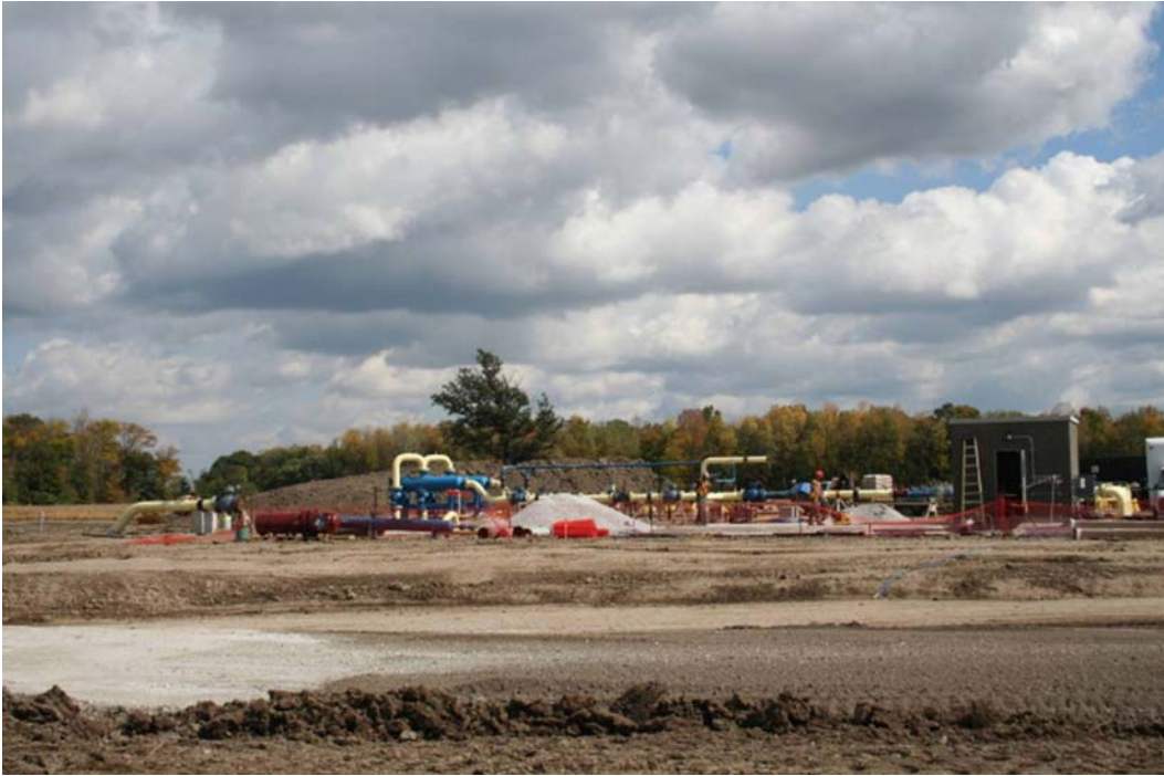
Natural gas pressure control and metering facility.
