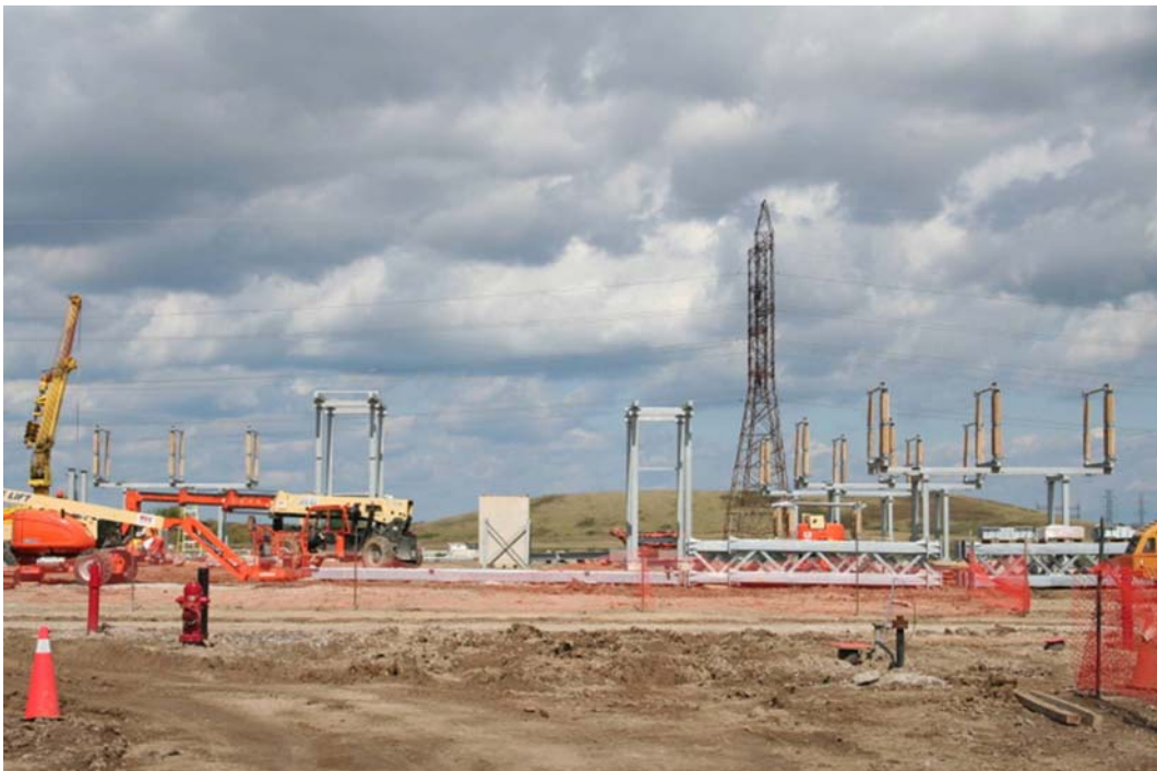
Switchyard for interconnection with the Hydro One 230kV transmission grid.
