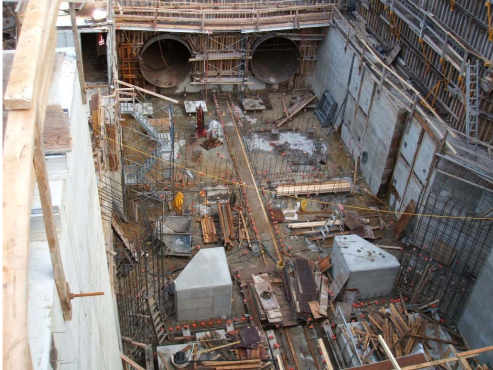
A view of the “Y” bifurcation leading to the yet to be installed power generating units.
