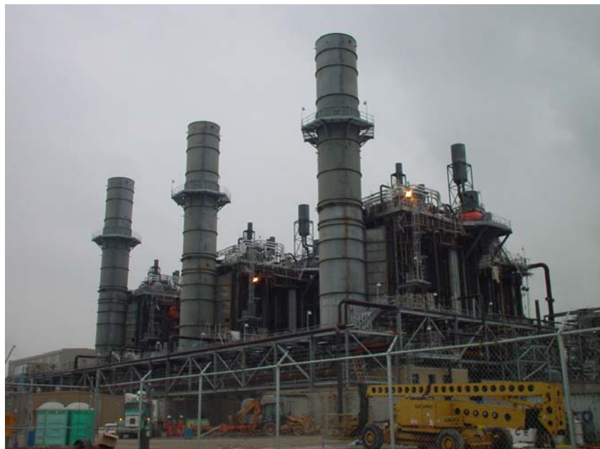
A view of the three generating units.
