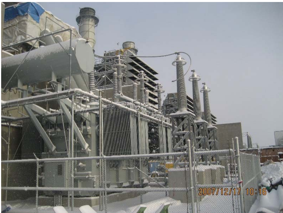
Generator step up transformers.
