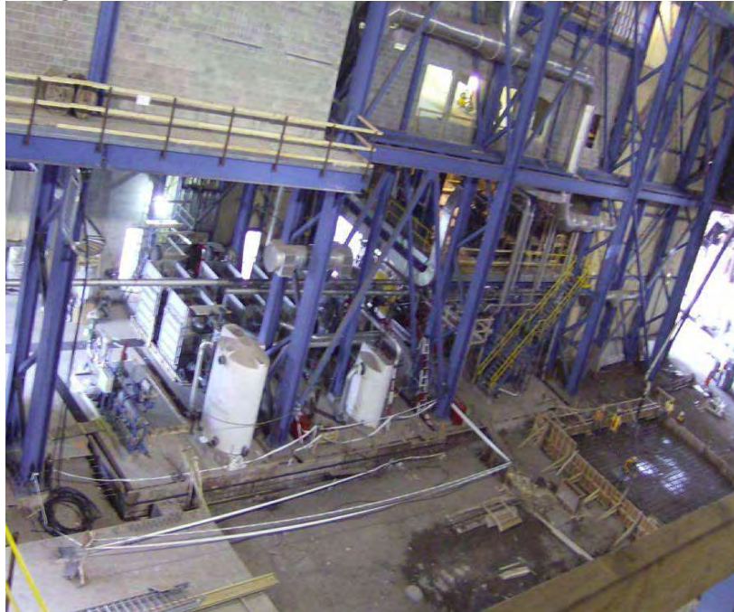
Water treatment plant installation at Algoma Energy Cogeneration site
