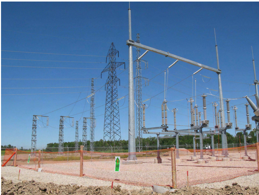
A section of the substation for the Enbridge Wind Farm has been energized and is being fenced off
