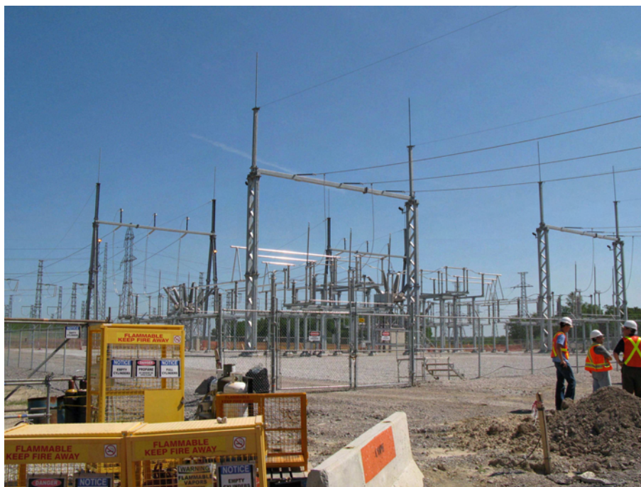
The substation at St. Clair Energy Centre is substantially completed
