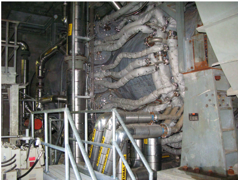
Insulation blankets have been installed at the combustion turbine at Greenfield Energy Centre
