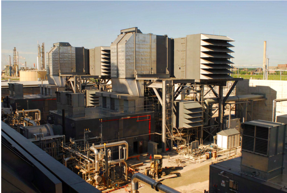
Air intake for two of the combustion turbine generators at the Greenfield Energy Centre
