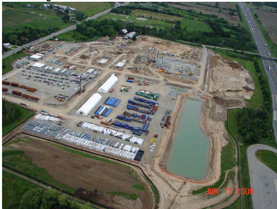
Aerial view of the Halton Hills Generating Station
