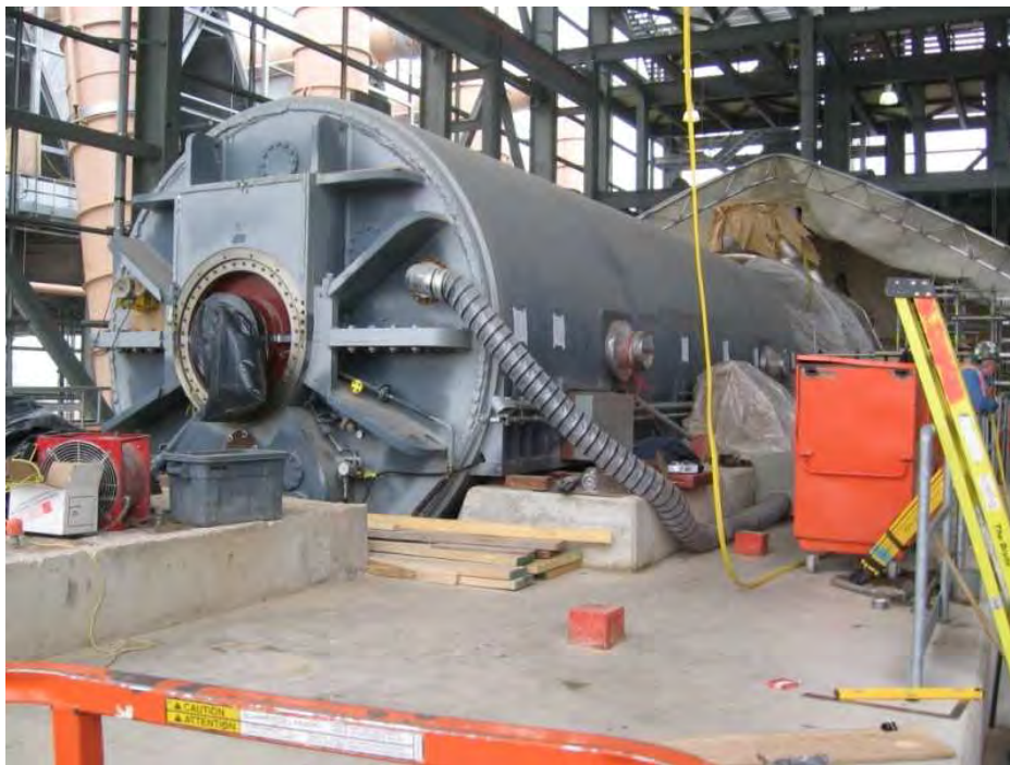
Steam turbine set on its foundation at Goreway Station
