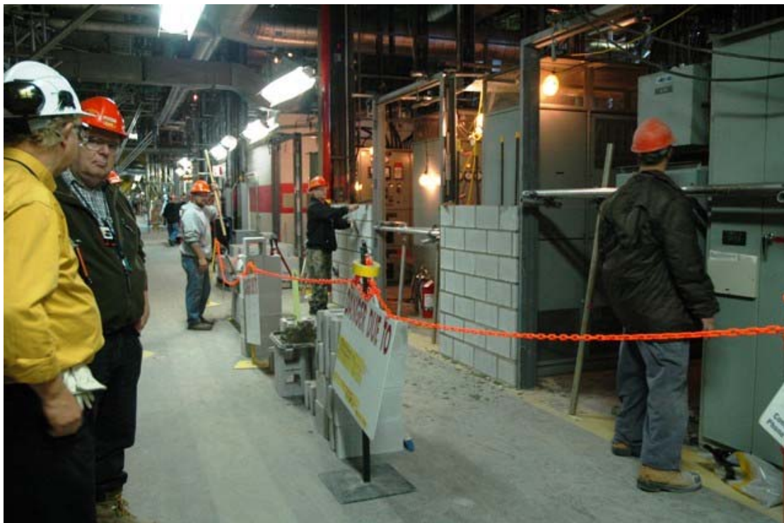
The power conversion rooms at Bruce A Units 1 and 2.
