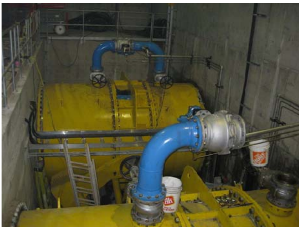
Butterfly inlet valves installed at the Umbata Falls Hydroelectric Project
