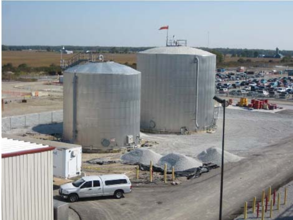
Demineralized and raw water tanks at the St. Clair Energy Centre
