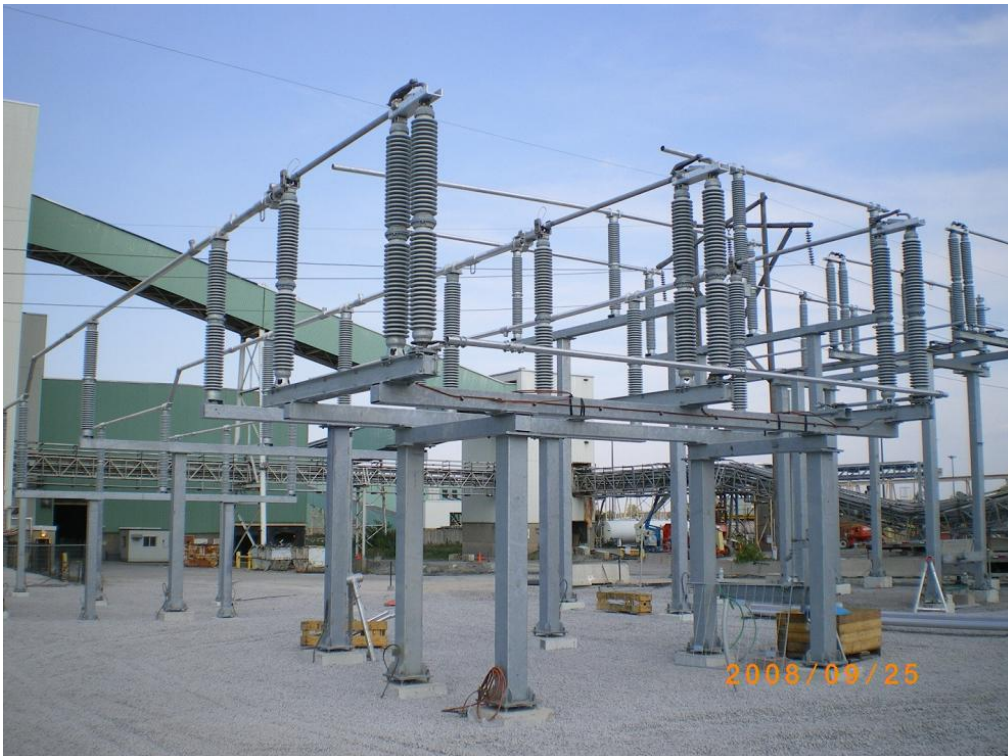
Host facility switchyard at the Thorold Cogeneration Project
