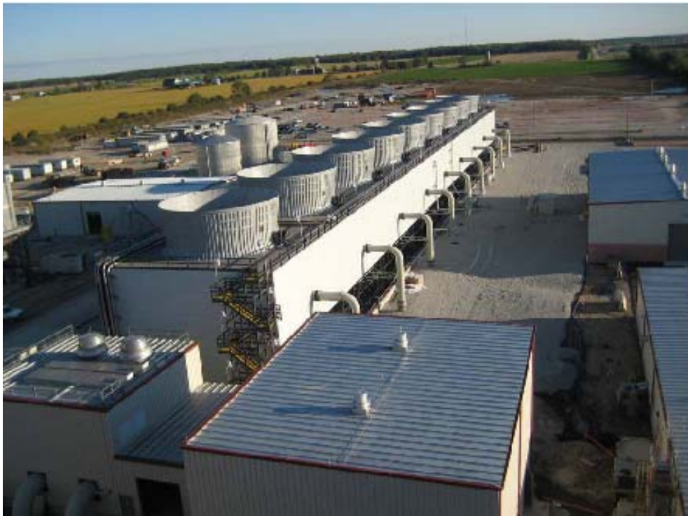
Cooling towers are in place at the St. Clair Energy Centre
