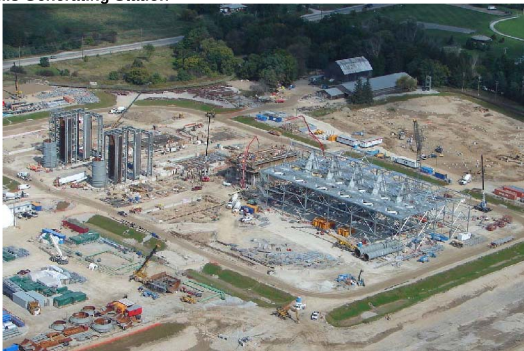
Aerial view of the Halton Hills Generating Station
