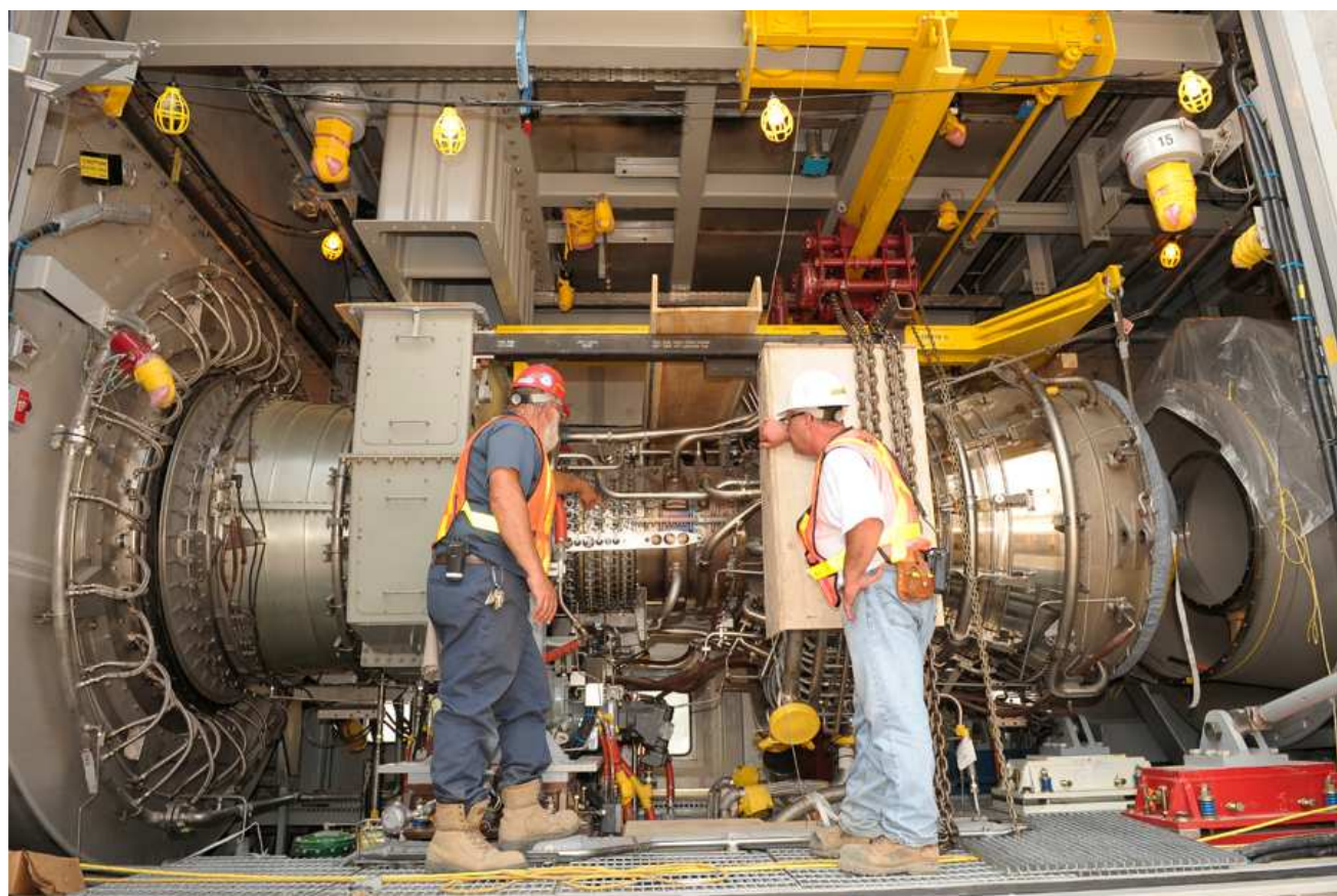
Inside the gas turbine generator at the East Windsor Cogeneration Centre
