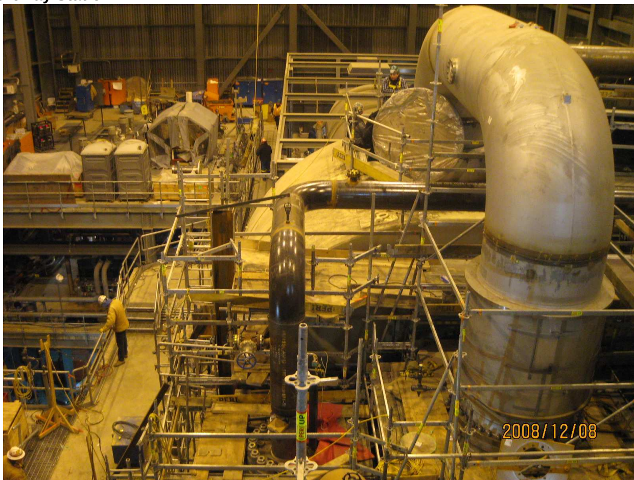
Steam turbine with blow piping at the Goreway Station
