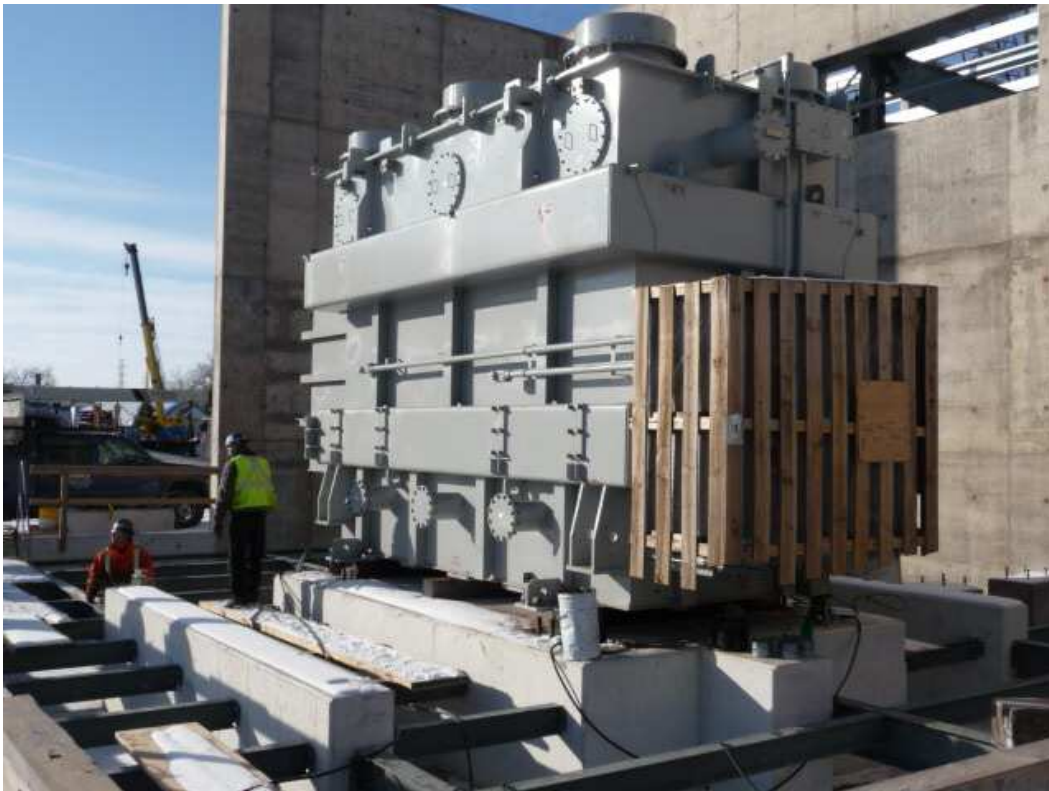
Transformer at the Thorold Cogeneration Project
