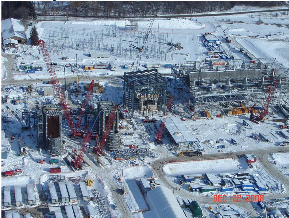
Aerial view of the Halton Hills Generating Station from the west
