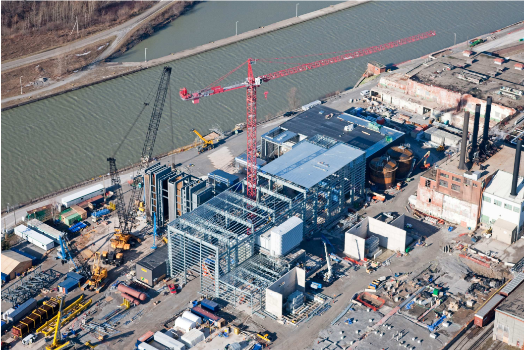
Aerial view of the Thorold Cogeneration Project
